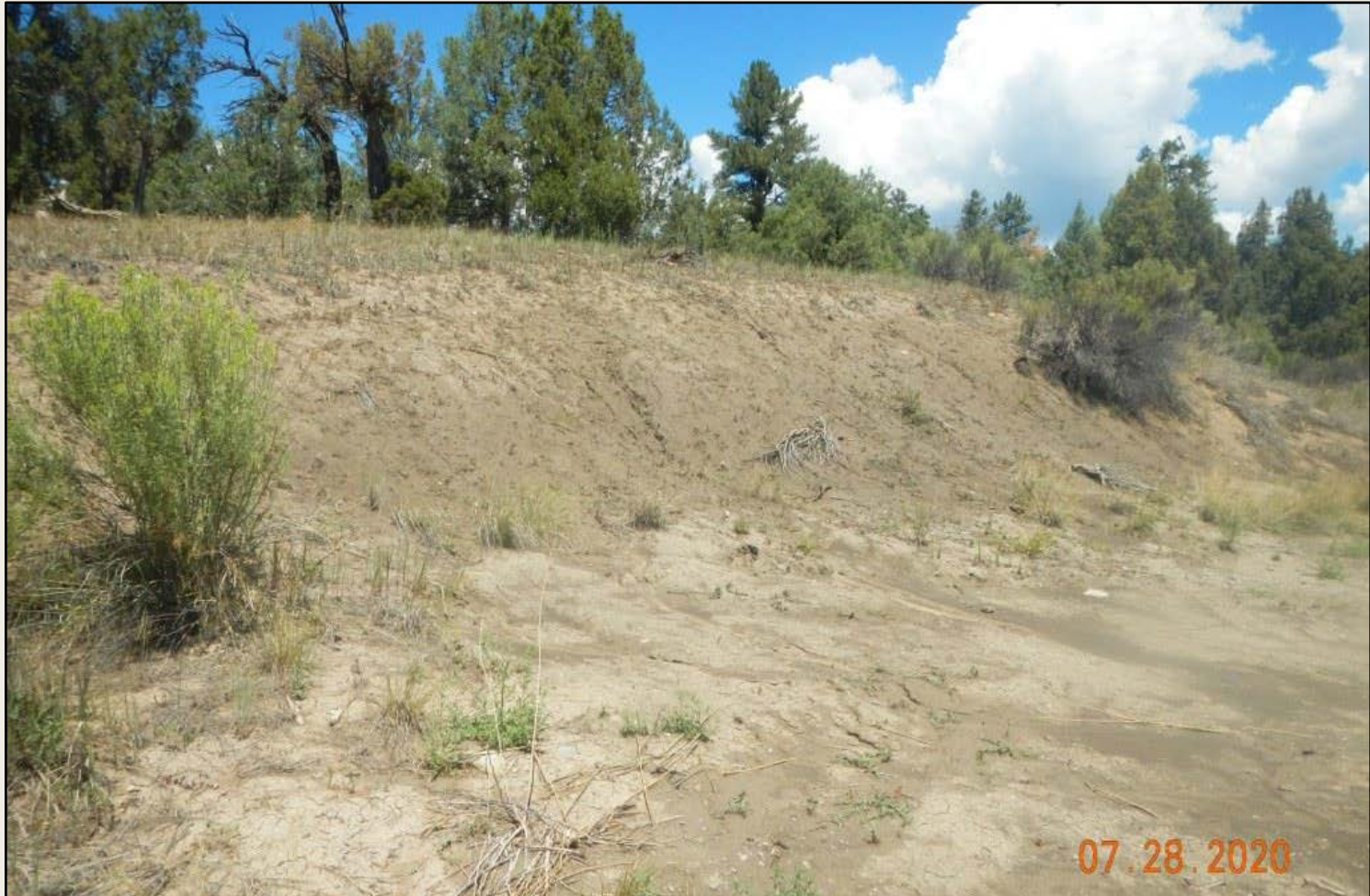
Photo 3. View of the western project area, cut-slope is not contoured or stabilized, as sediment deposition observed at the toe of the slope.
