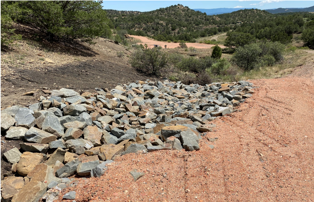
Photo 4. The area of erosion along the road has been stabilized with rock rip/rap.
