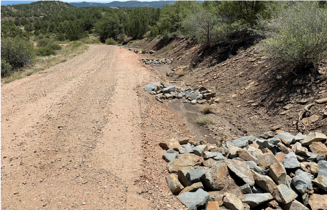
Photo 5. Facing southeast along the opposite side of the road. Rock check dams have been repaired.
