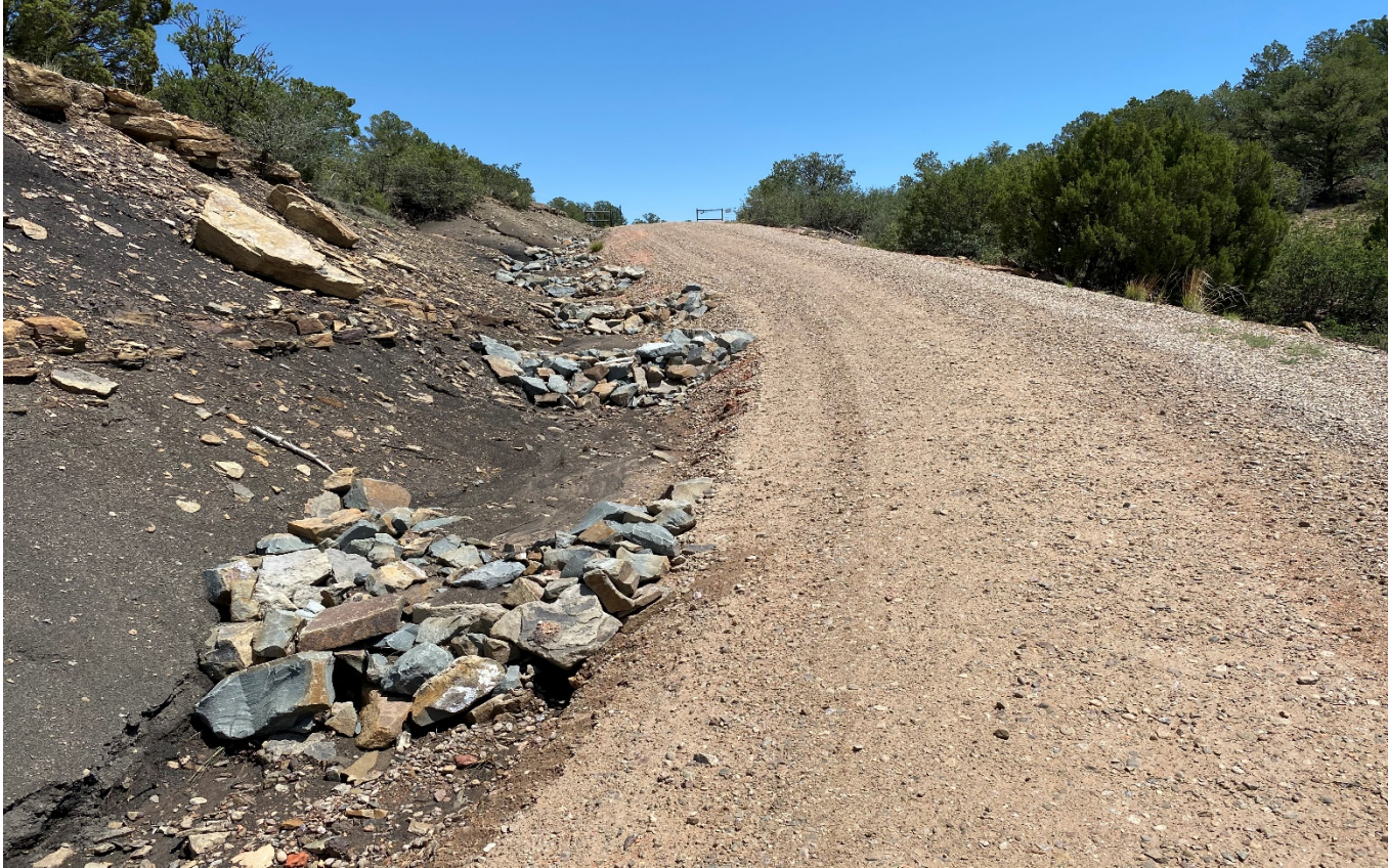
Photo 3. The rock check dams have been installed and repaired. The check dams will need to be maintained.
