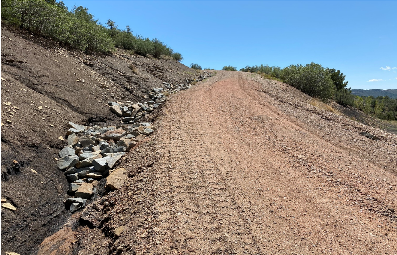
Photo 1. Facing southeast along the access road. Rock check dams have been installed along the side of the road where erosion was occurring.
