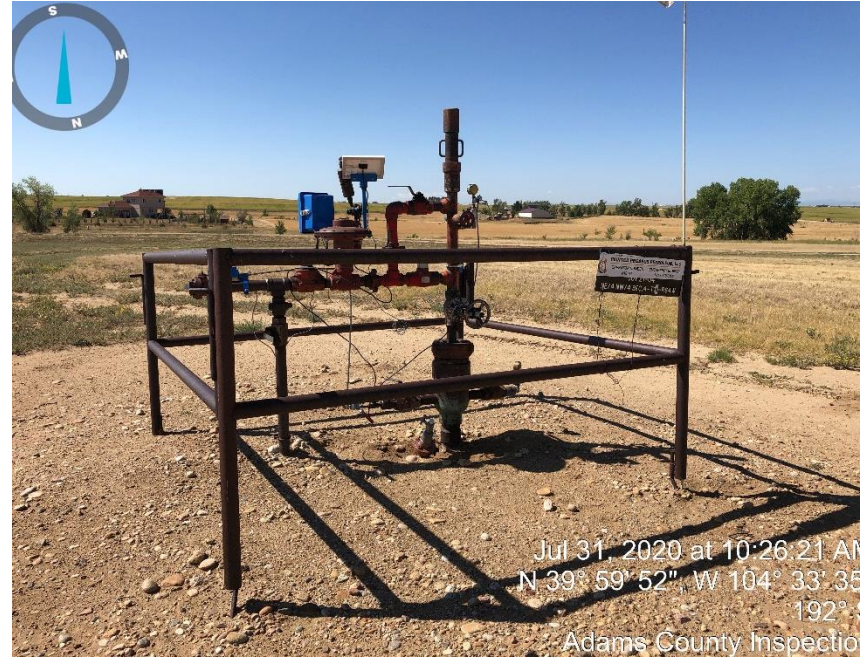
Photo #4 Well Head.
