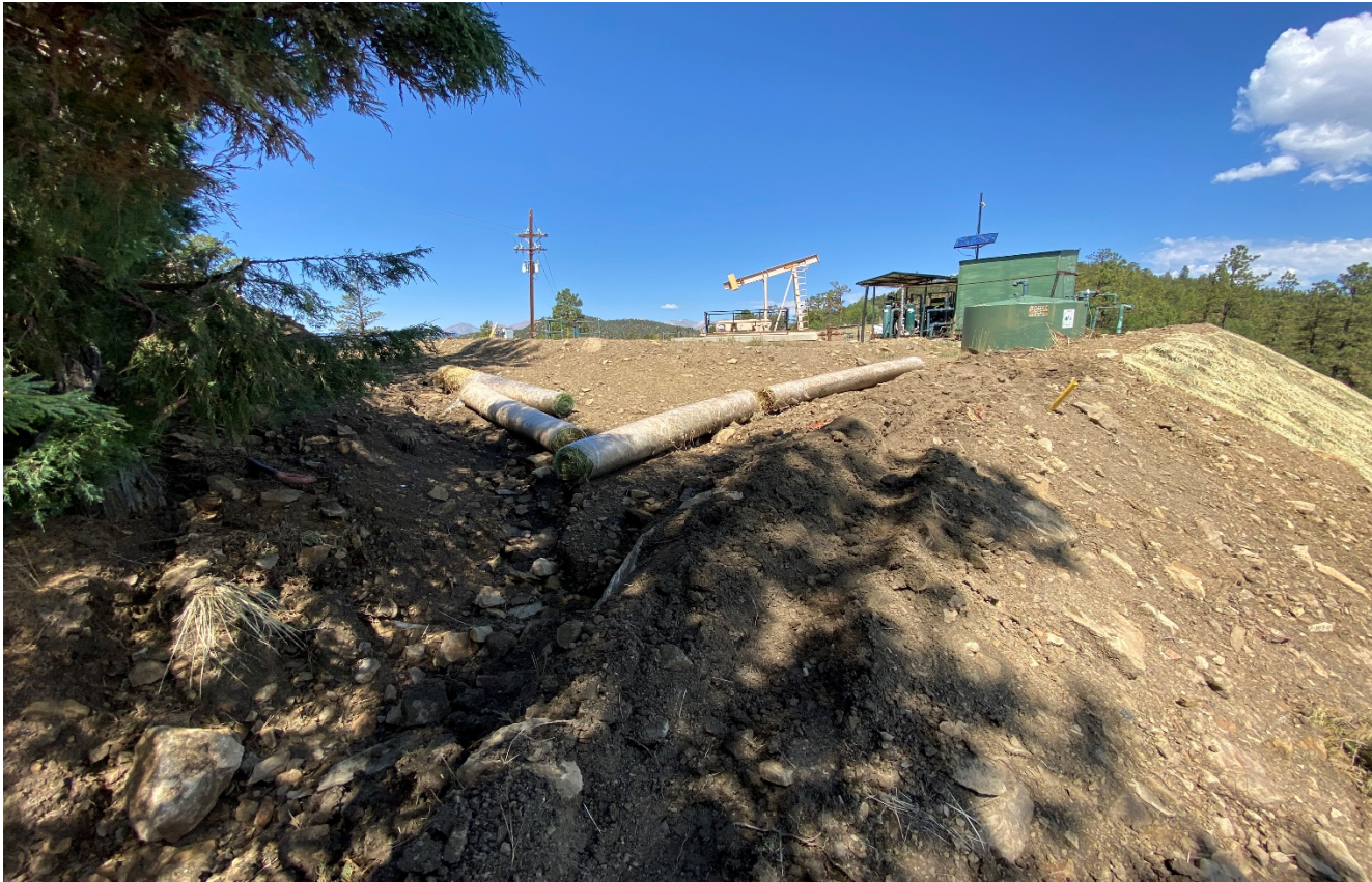
Photo 5. Southeast corner facing toward the location. It appears work is still in progress installing straw blanket.
