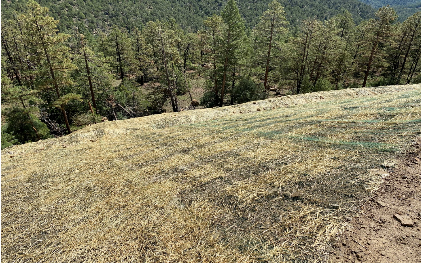
Photo 3. Facing down toward the fill slope. This area which had sloughed off has been resloped and temporarily stabilized with straw blanket.
