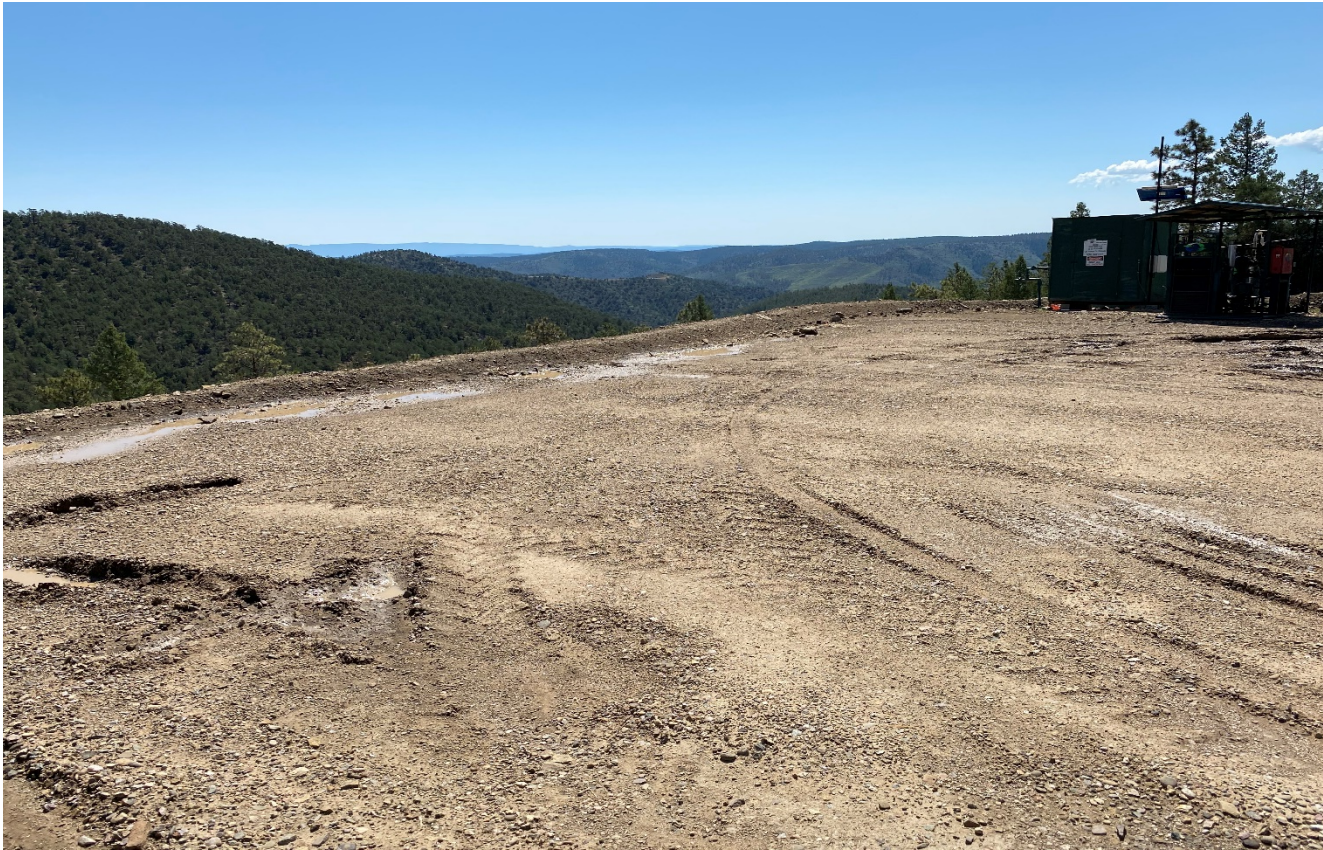
Photo 2. Facing southeast at the location. This area of the location appears to have been stabilized and the fill slope is resloped.
