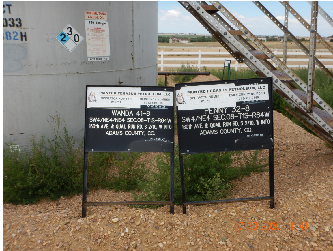
Photo 3. Photo taken from the tank battery, facing West. Photo illustrates Operator signs and which wells the tank battery services.
