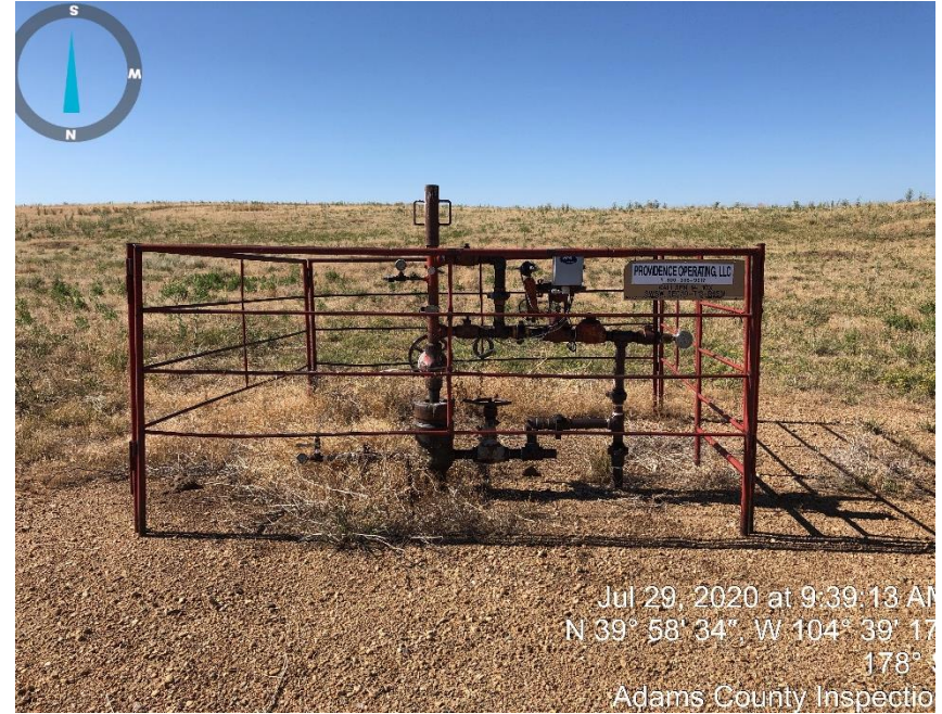
Photo #4 Well Head.
