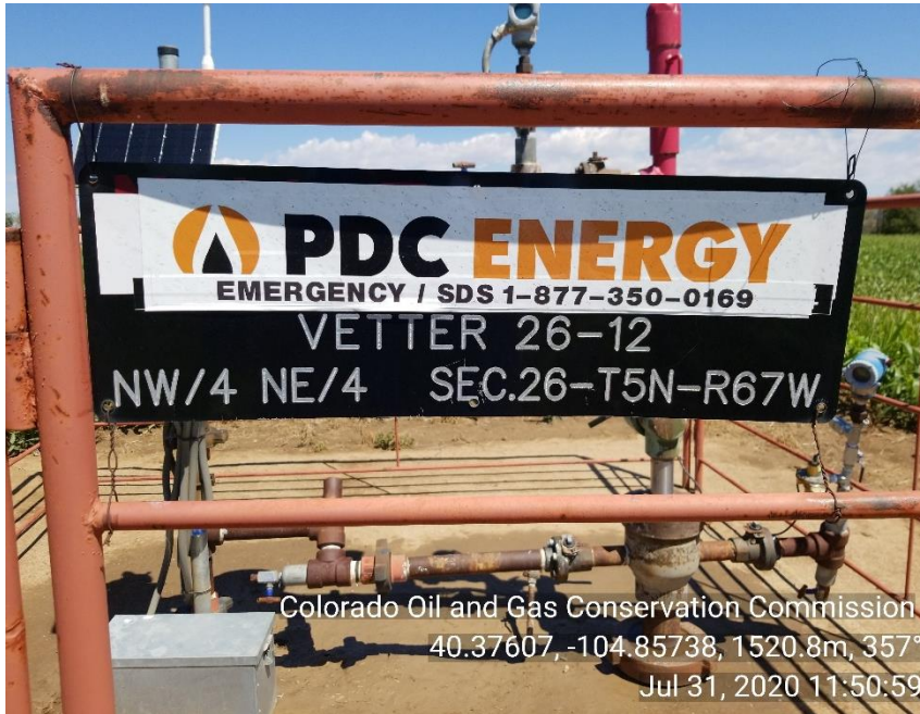
Photo 1: Wellhead Sign; emergency # installed
