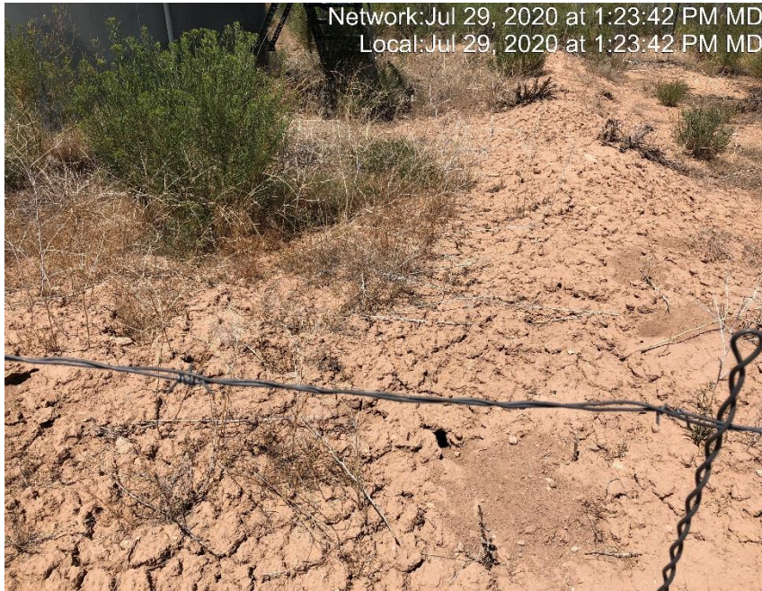
Photo #1641 Tank berm has eroded.
