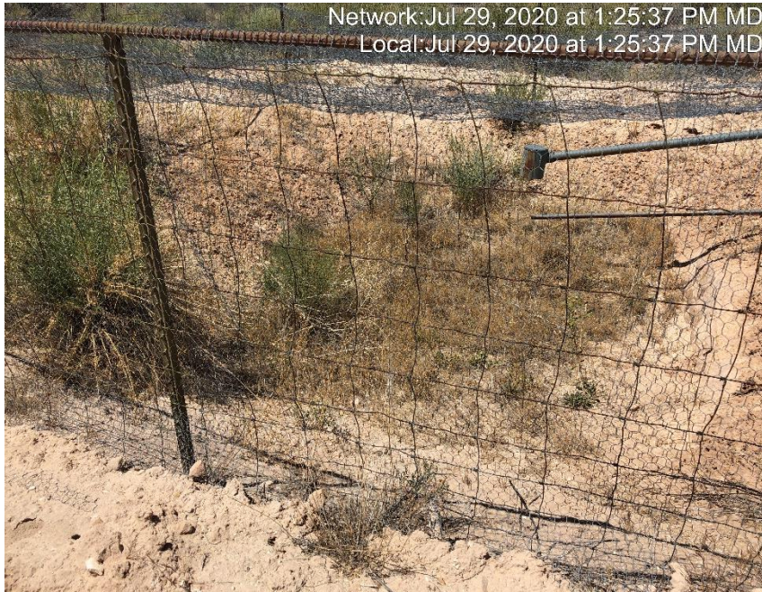
Photo #1643 Multiple places with debris on location.
