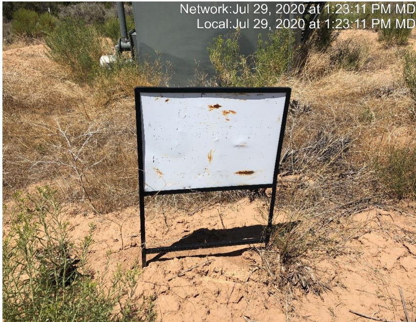
Photo #1639 Battery sign is weathered and not legible.
