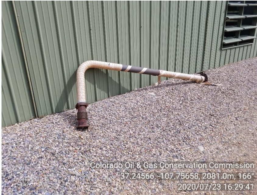
PHOTO 5: UNUSED EQUIPMENT (4" PIPE LEANING AGAINST SOUND WALLS). REMOVE UNUSED EQUIPMENT PER RULE 603.f. CA DATE 10-23-20.
