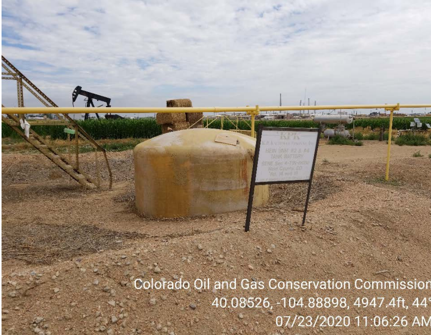
Photo 1 – Battery location sign
