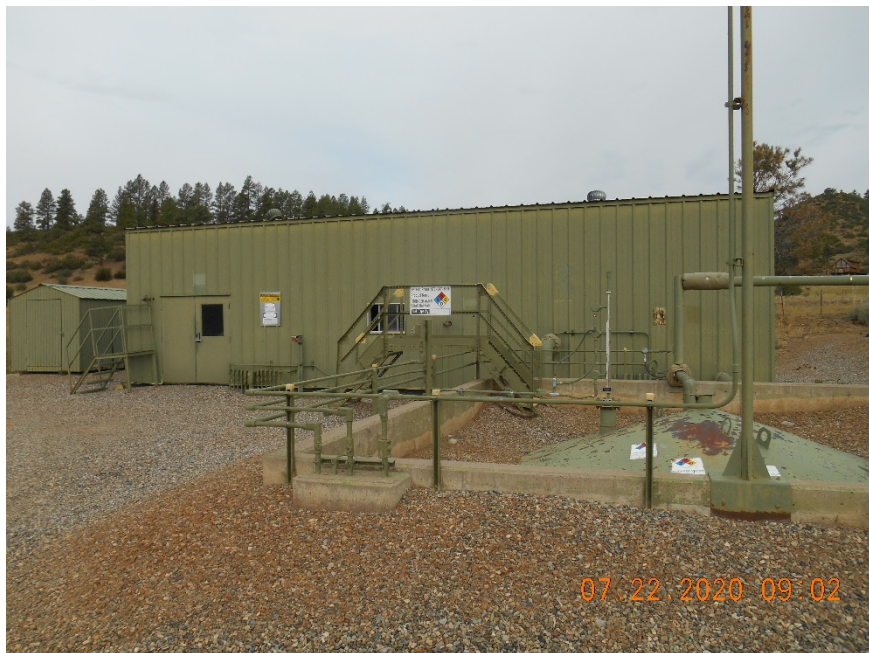
Pump housing. Partially buried blowdown tank
