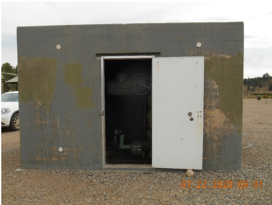
Injection wellhead inside housing
