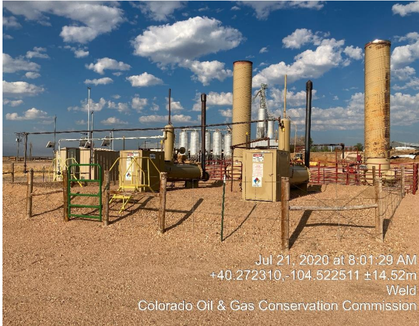
Photo #2 Separators, ECD's & Meter Runs
