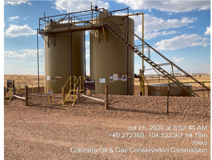
Photo #3 Tank Battery
