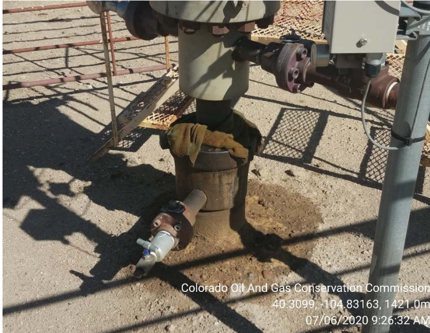
Bradenhead packing leak and stained soil on 7/6/2020
