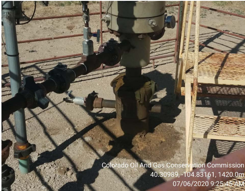
Bradenhead packing leak and stained soil on 7/6/2020
