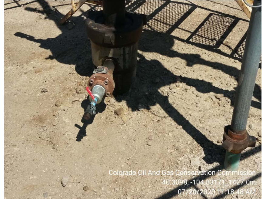
Bradenhead packing leak and stained soil on 7/20/2020
