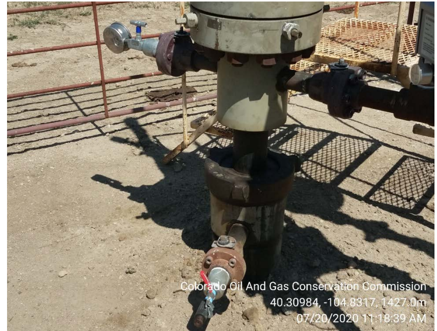
Bradenhead packing leak and stained soil on 7/20/2020
