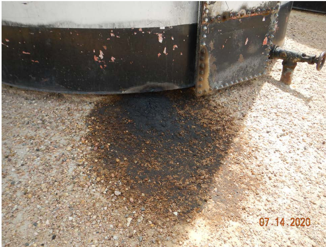
Photo # 6 – Northwest side of northern tank, oil stained soil and tank leaking from corrosion holes
