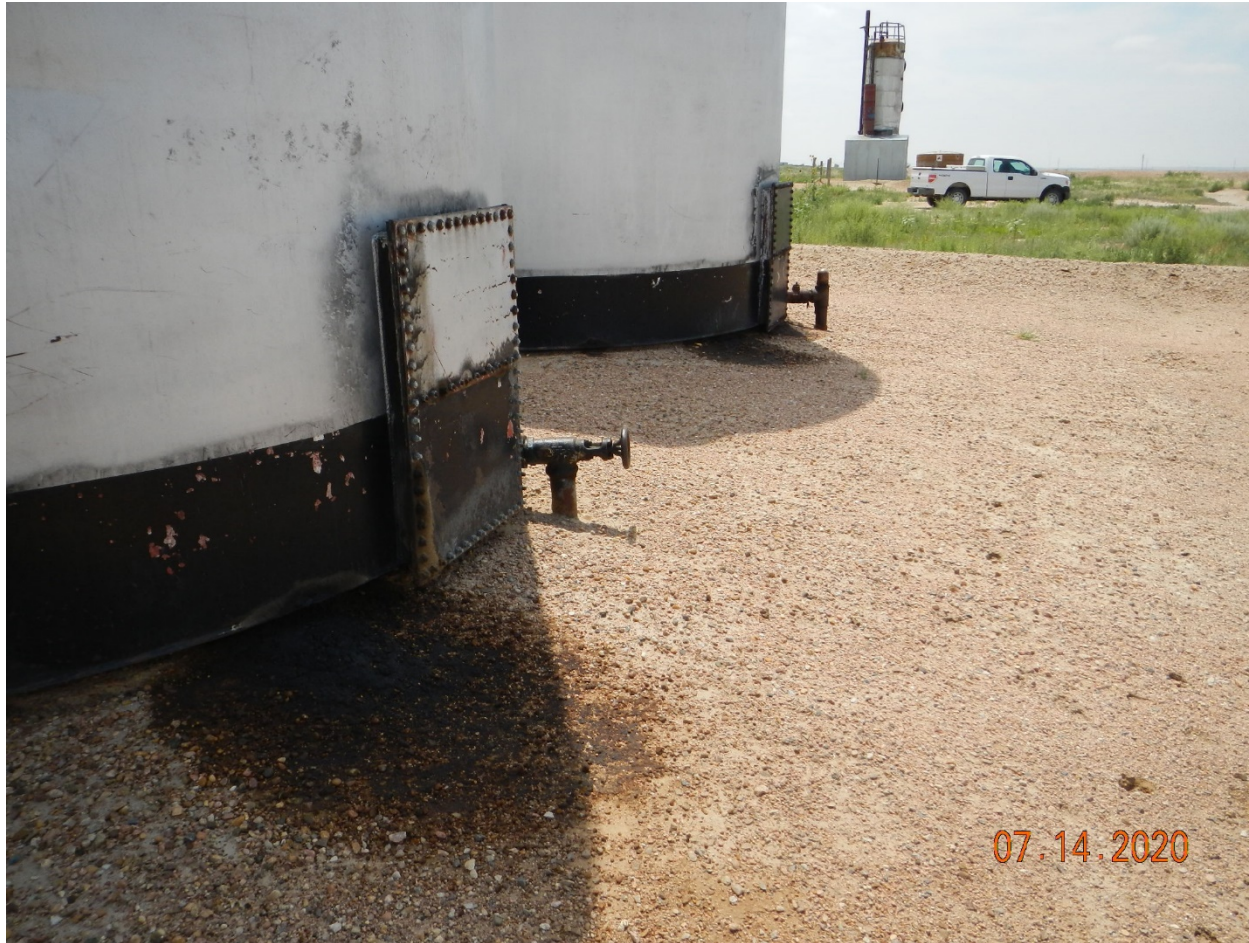
Photo # 7 – Northwest side of northern tank, oil stained soil and tank leaking from corrosion holes (also south tank)
