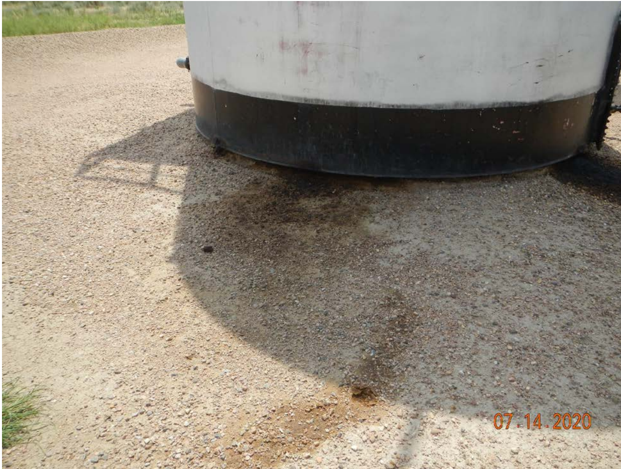
Photo # 5 – North side of northern tank, oil stained soil and tanks leaking from corrosion holes
