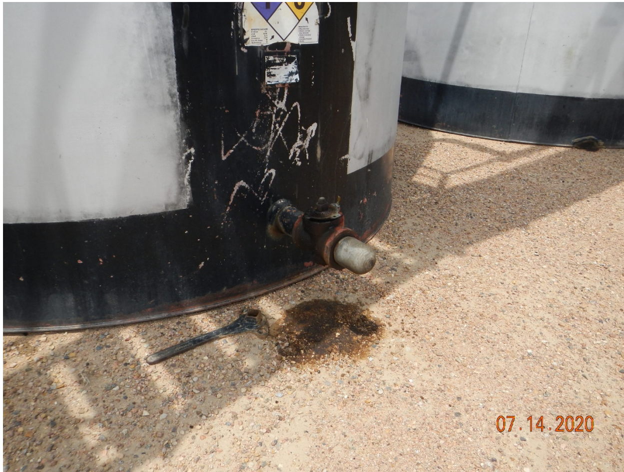
Photo # 3 – East side of tank battery, oily soil under valves and bottom of north tank
