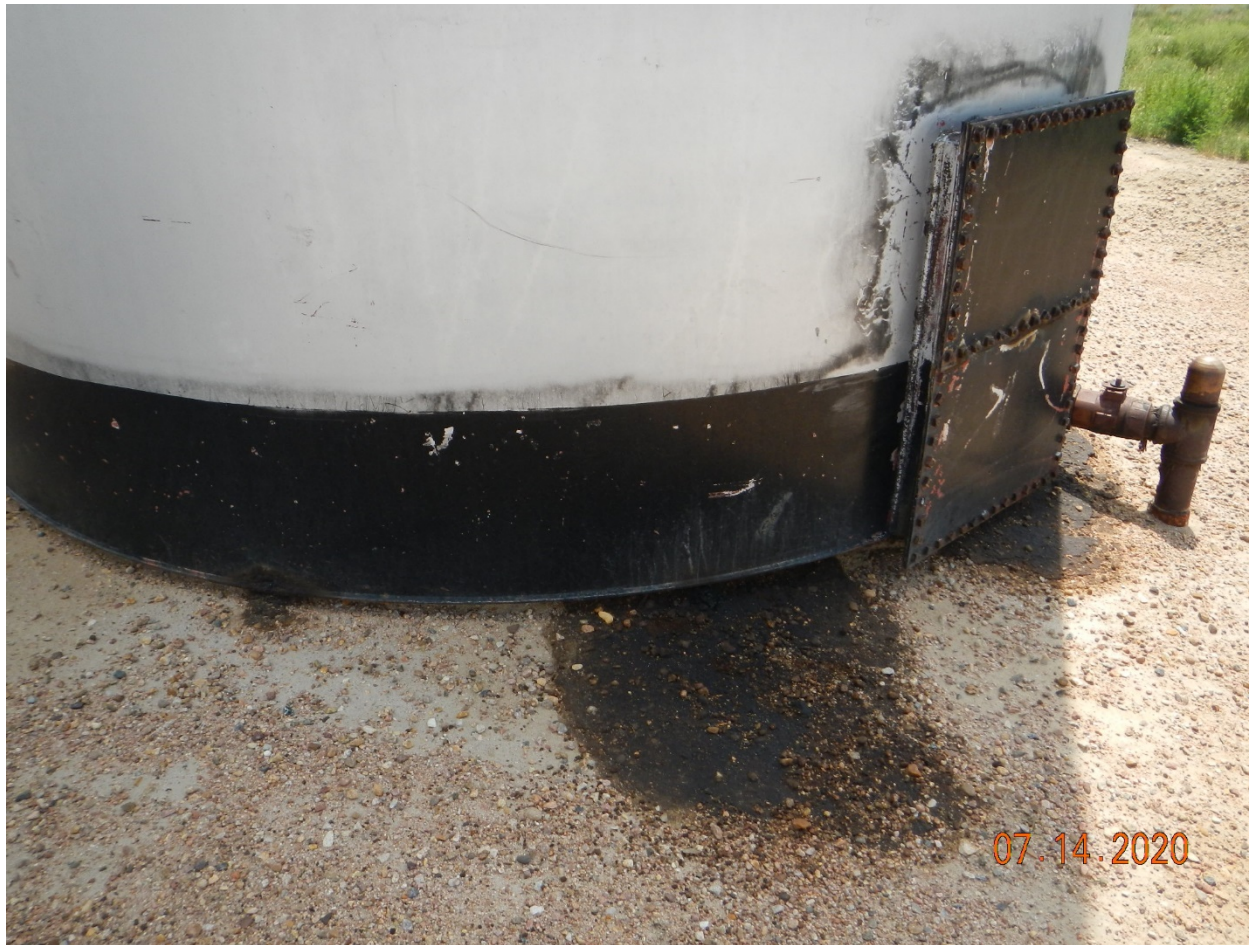
Photo # 8 – Northwest side of southern tank, oil stained soil and tank leaking from corrosion holes
