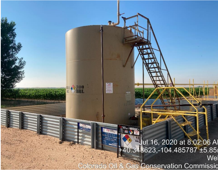
Photo #3 Tank Battery
