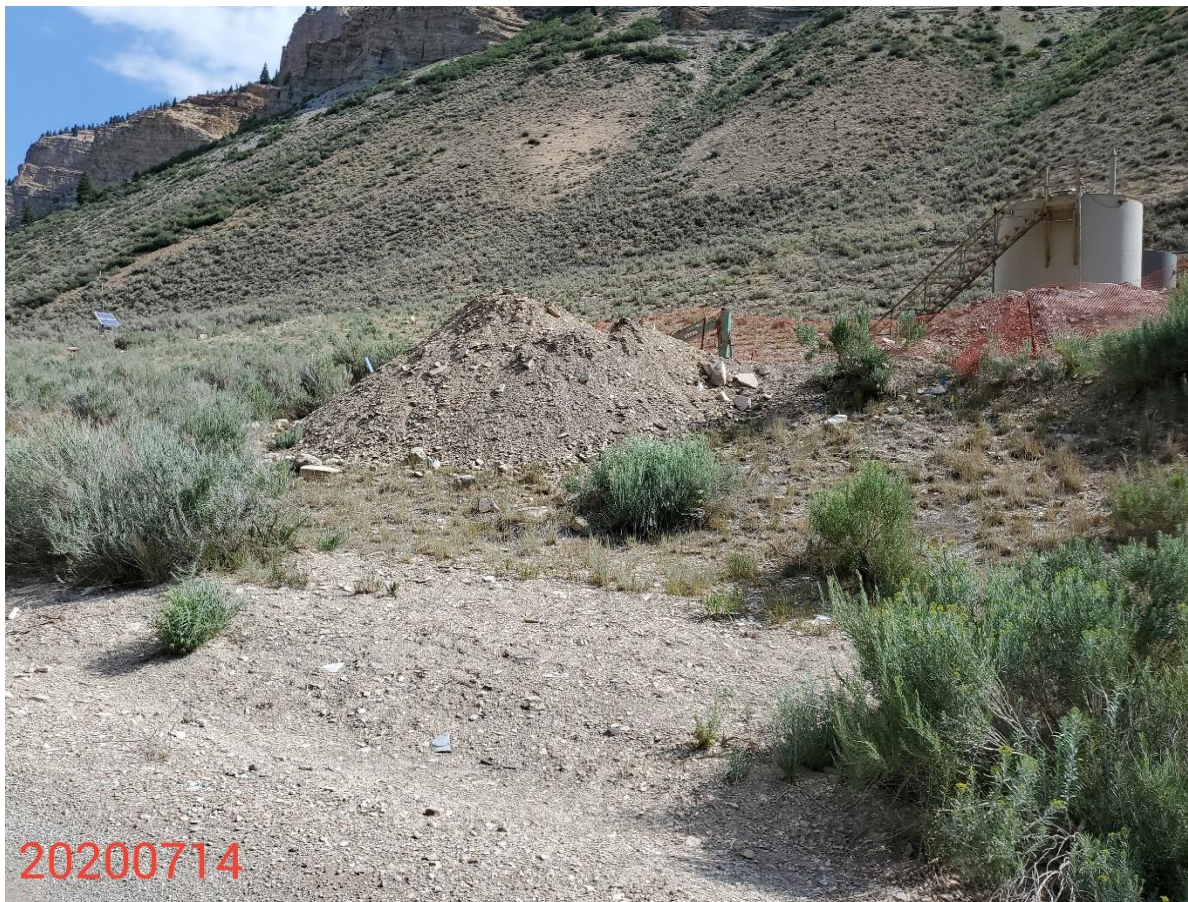
Photo 4: Photo taken from the west of the Location, facing northeast. Photo shows BMPs to prevent sediment transport from the soil stockpiles are missing or insufficient.
