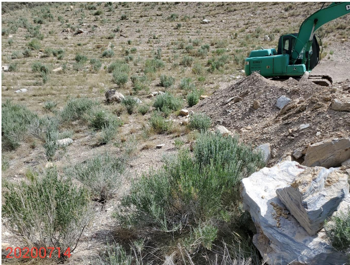
Photo 6: Photo taken from the north end of the Location, facing east. Photo shows BMPs to prevent sediment transport from the soil stockpiles are missing or insufficient.
