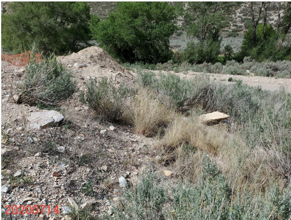
Photo 5: Photo taken from the north end of the Location, facing west. Photo shows BMPs to prevent sediment transport from the soil stockpiles are missing or insufficient.
