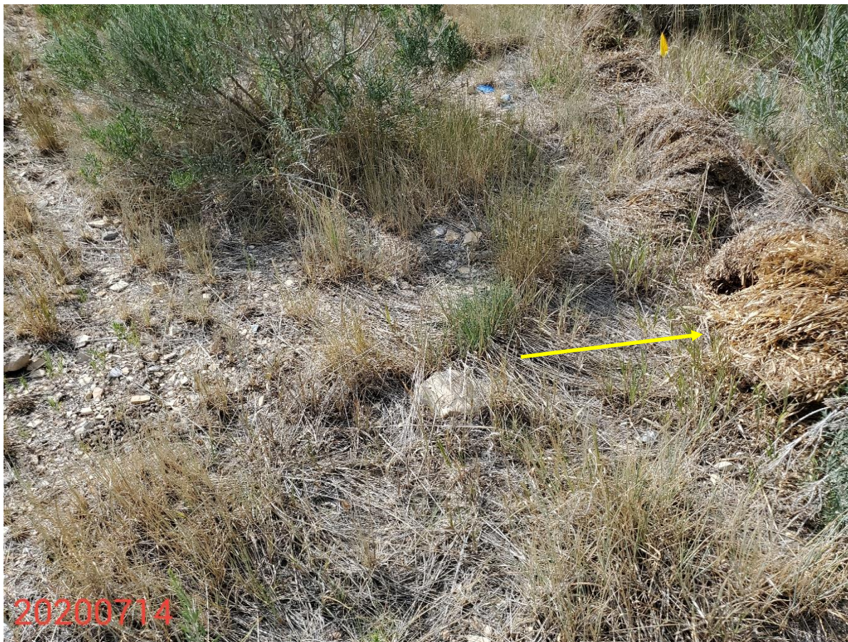
Photo 7: Photo taken with use of a west end of the Location. Photo shows straw hay bale BMPs along the west end of the Location is has not been maintained and is not in proper functioning condition.
