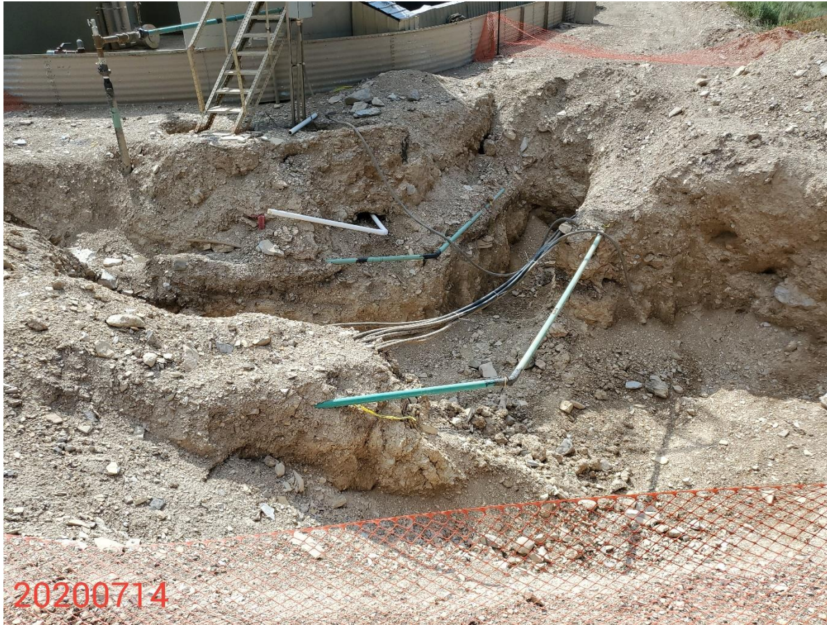
Photo 8: Photo taken from the northwest end of the Location. Photo shows excavated areas due to dumpline spill.
