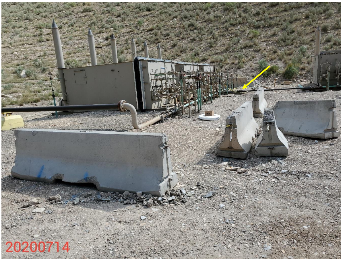
Photo 9: Photo taken from the northeast end of the Location, facing east. Photo shows equipment and 2 nd area of the Location where excavation activities are evident.
