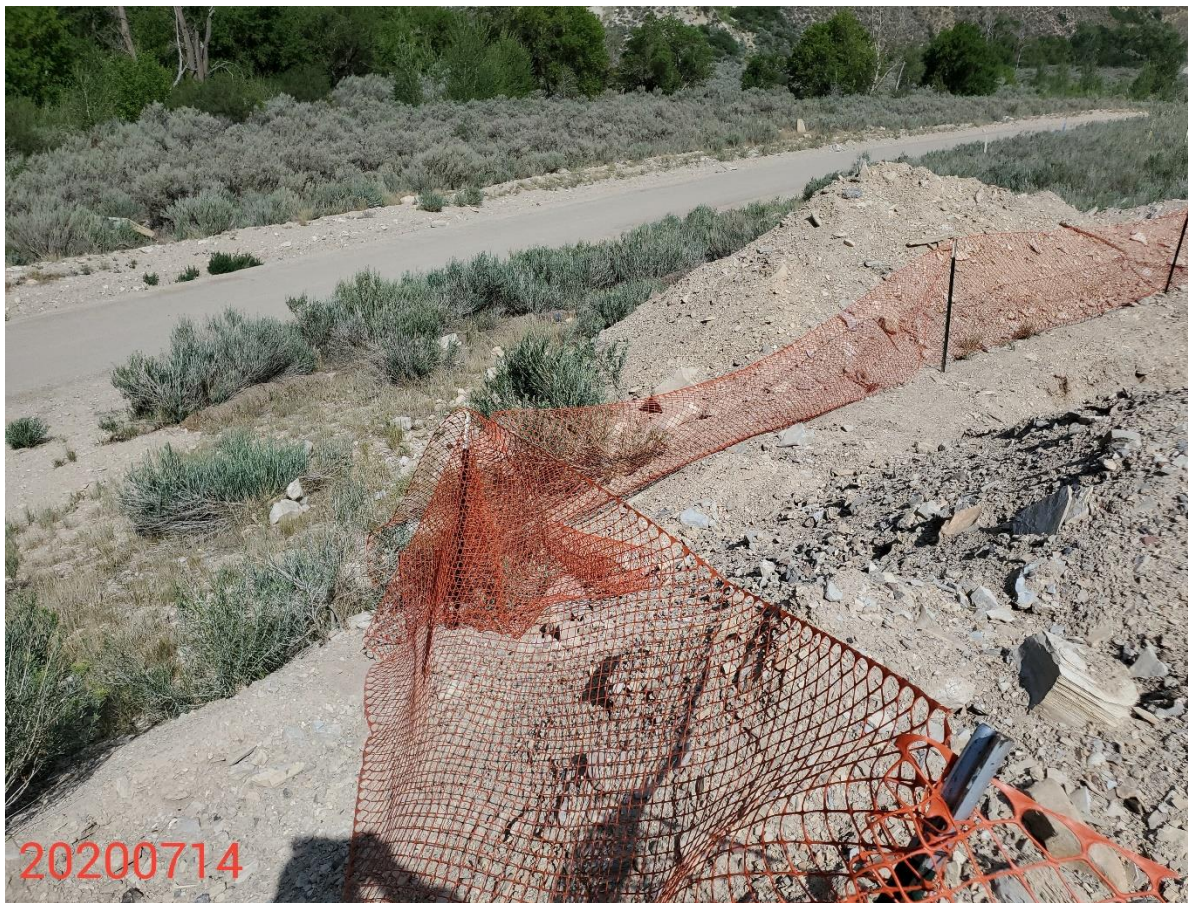
Photo 2: Photo taken from the northwest end of the Location, facing northwest. Photo shows excavated areas due to dumpline spill, and the soil stockpiles.
