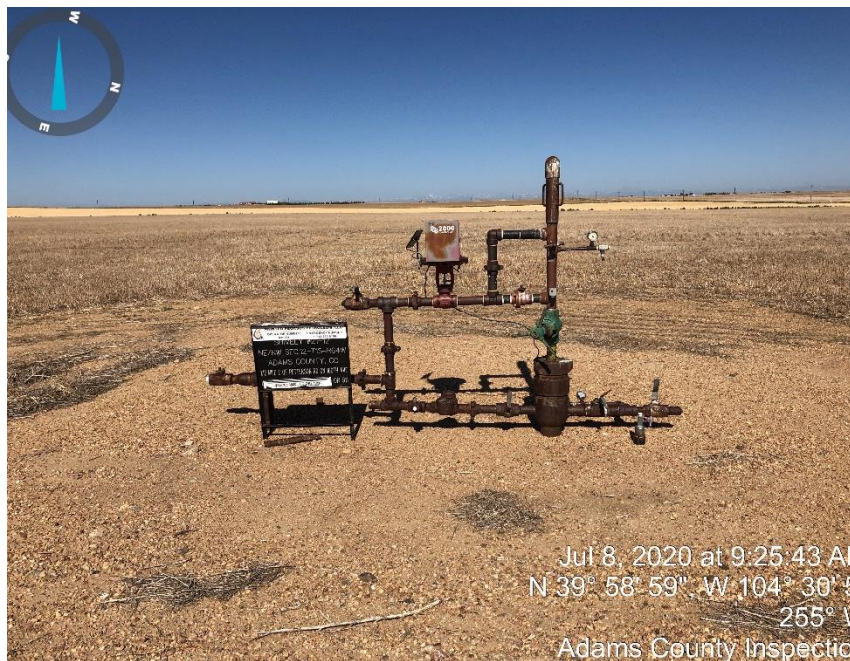
Photo #5 Well head.
