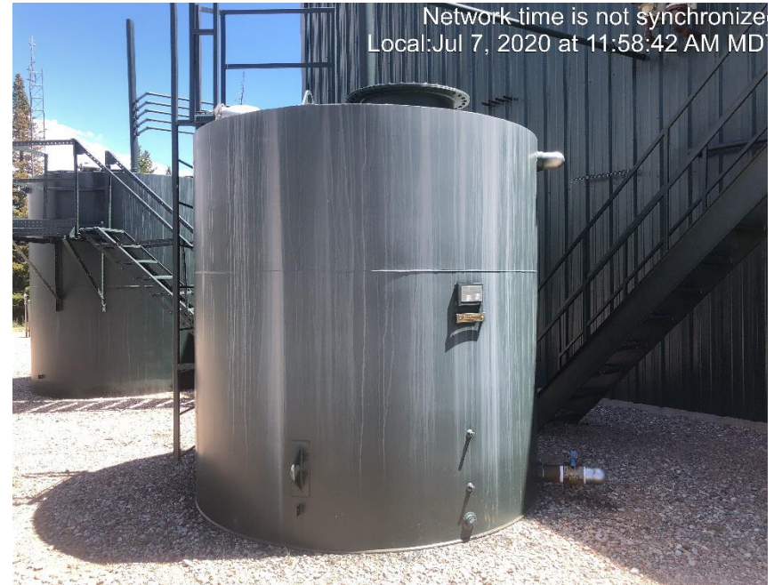
Photo #1463 Multiple tanks missing required information
