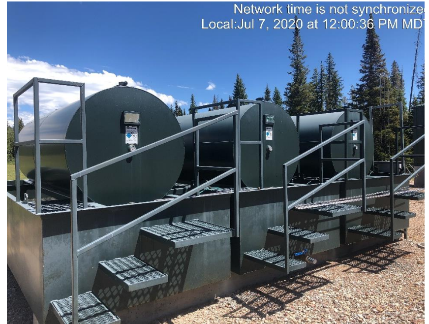
Photo #1465 Multiple tanks missing required information
