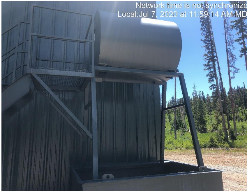
Photo #1464 Multiple tanks missing required information
