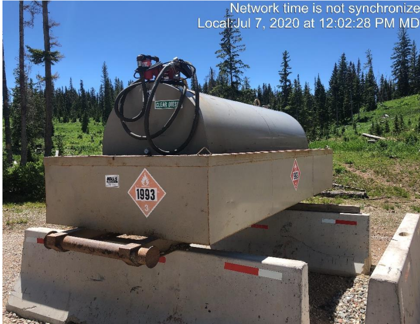
Photo #1466 Multiple tanks missing required information
