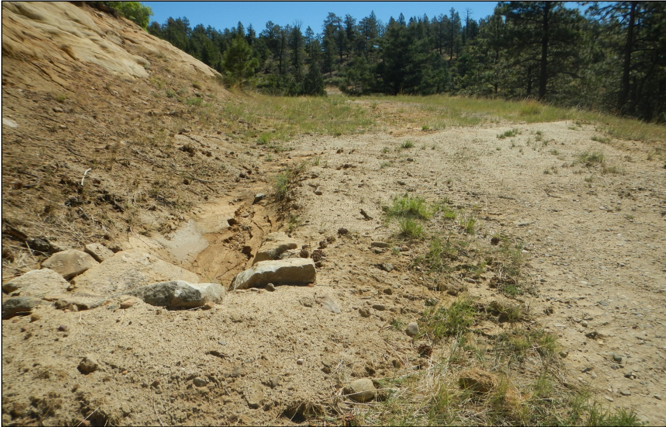
Photo 2. The culverts along the access road have been cleaned out and repaired..
