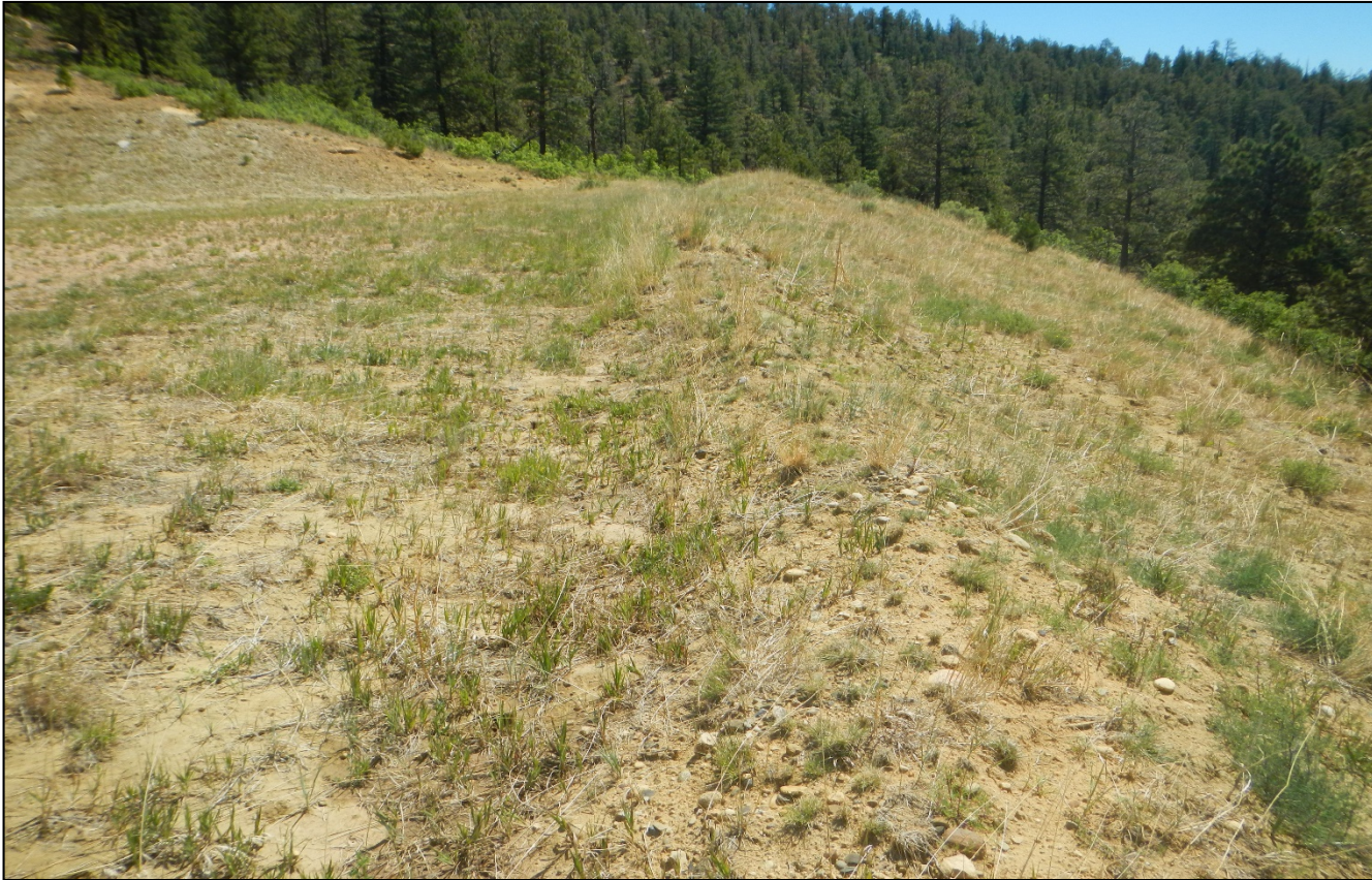
Photo 7. Facing east along the fill slope. Vegetation is well established along fill slope.
