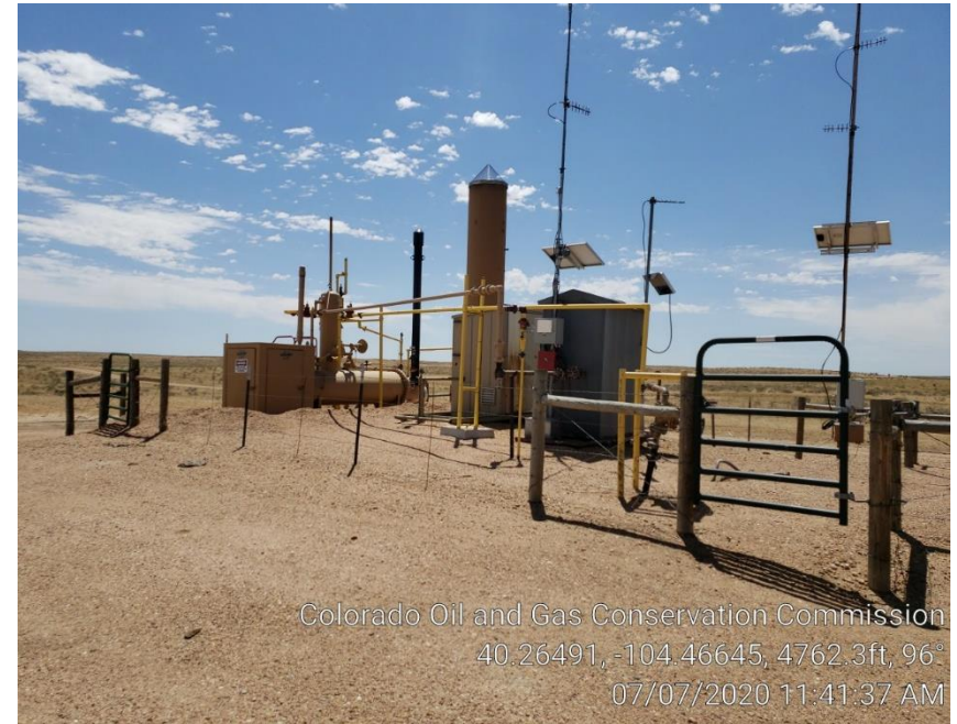
Photo #2 Separator, ECD & Meter Runs
