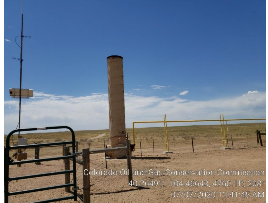
Photo #4 ECD for Tanks
