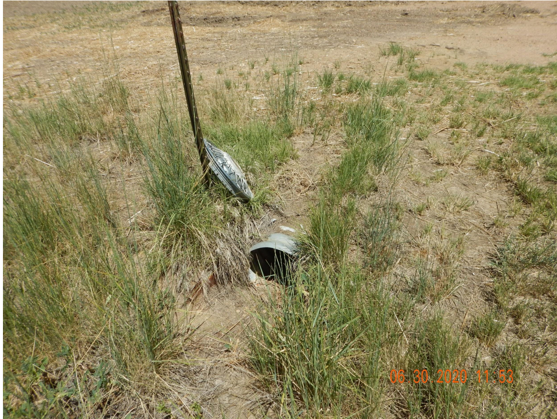
Photo 2. Photo taken from the entrance of location, facing North. Photo illustrates a culvert that has not been removed. Operator may need to remove that culvert or provide surface owner documentation.
