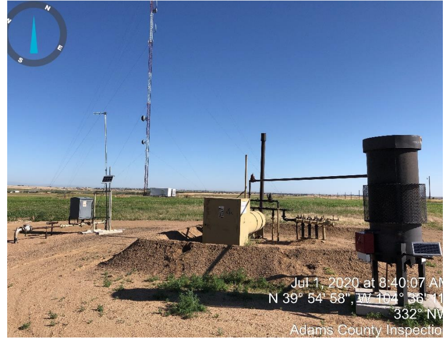
Photo #2 ECD, meter run and Separator
