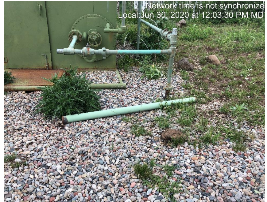
Photo #1441 Multiple places with unused equipment.
