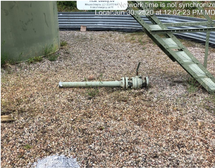
Photo #1439 Multiple places with unused equipment.
