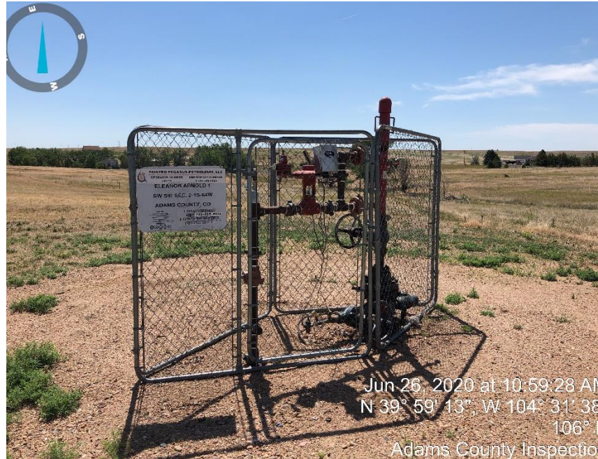
Photo #1 Well head.
