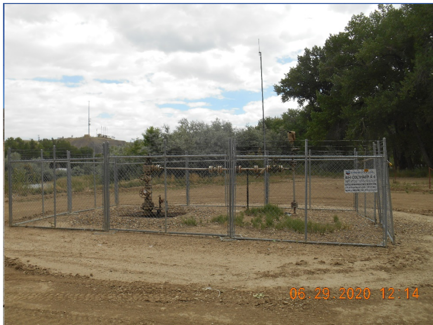
Injection wellhead. Temporarily Abandoned
