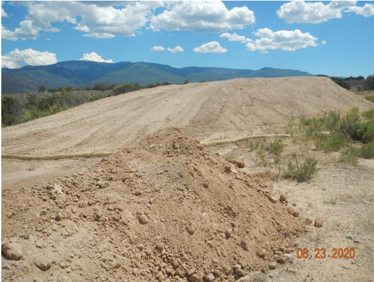
Photo#2: Topsoil Stockpile.
