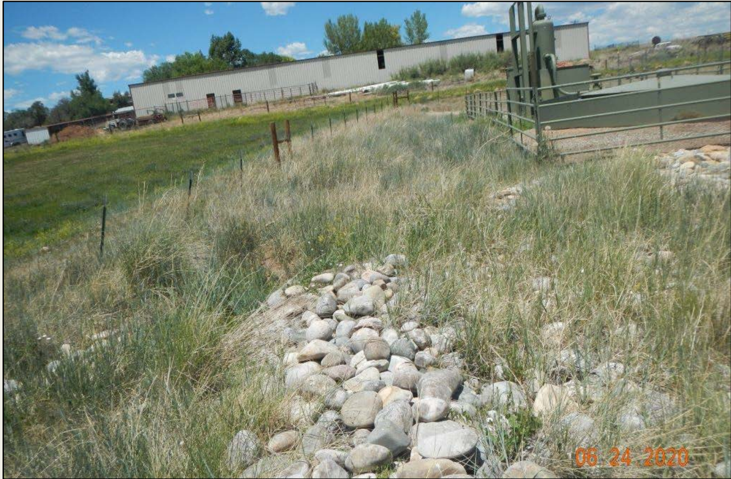
Photo 4. View of the western fill slope from the southwestern corner facing northward. Revegetation is progressing here with grasses such as western wheatgrass and crested wheatgrass. Weeds need to continue to be managed.
