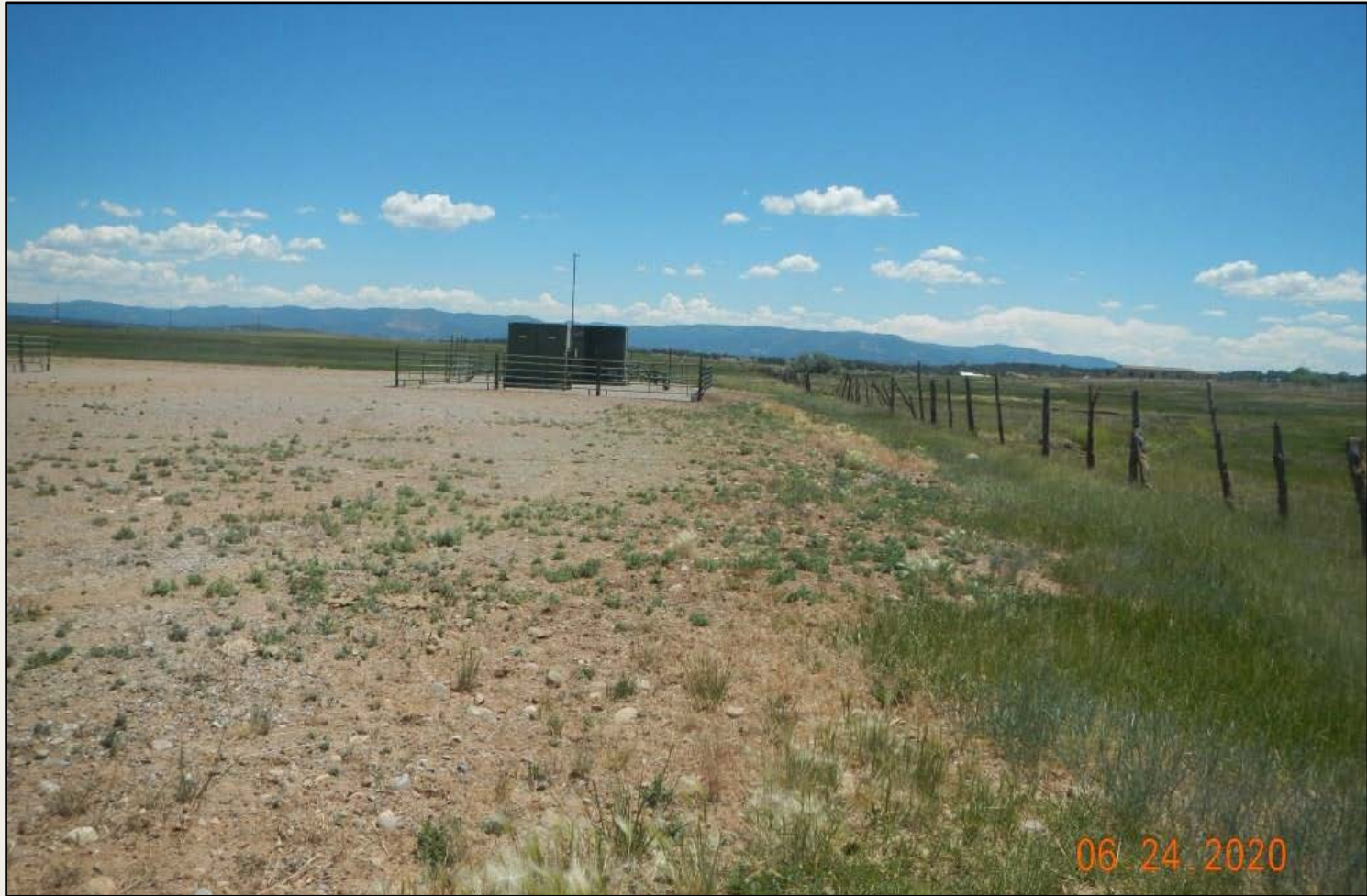
Photo 2. View of the southern fill slope from the southwestern corner facing eastward. Revegetation is progressing with irrigated pasture grasses.
