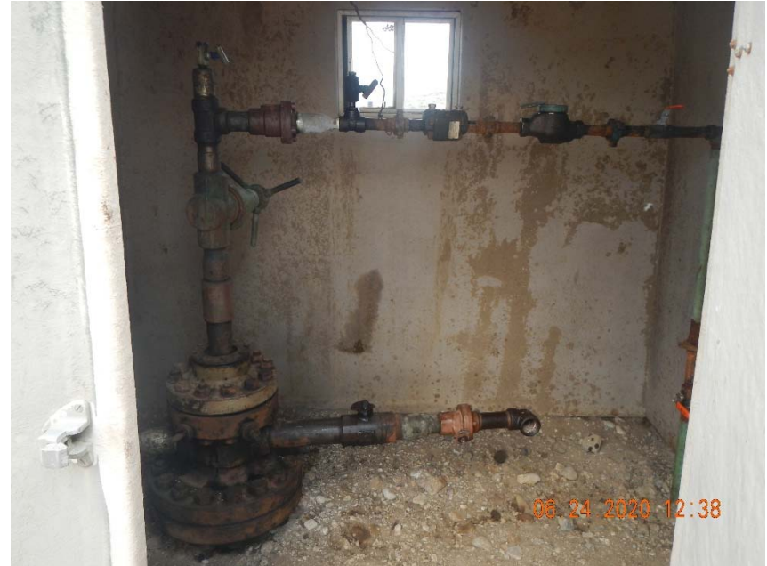
Photo 2. Photo of wellhead inside housing.
