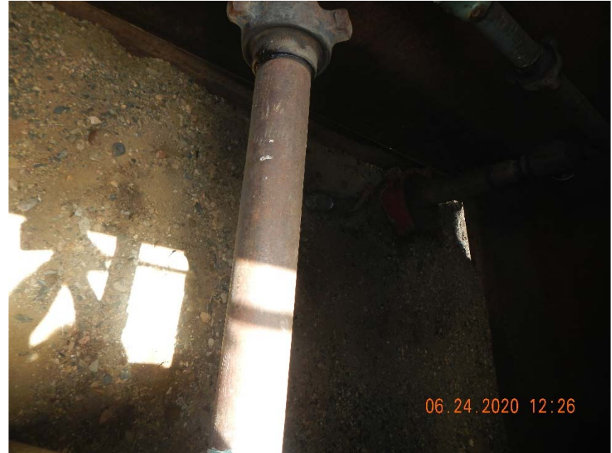
Photo 2. Photo of wellhead inside housing.
