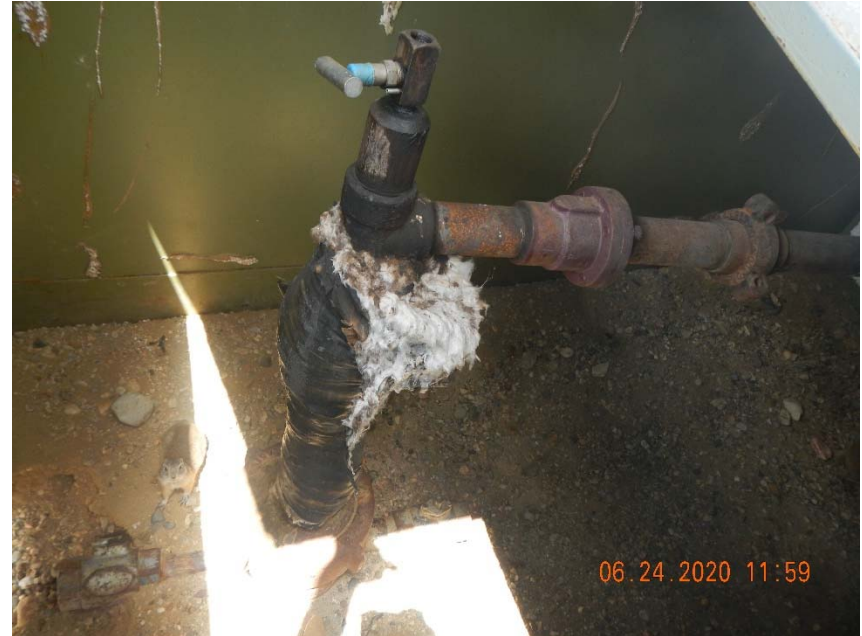
Photo 2. Photo of wellhead inside housing.
