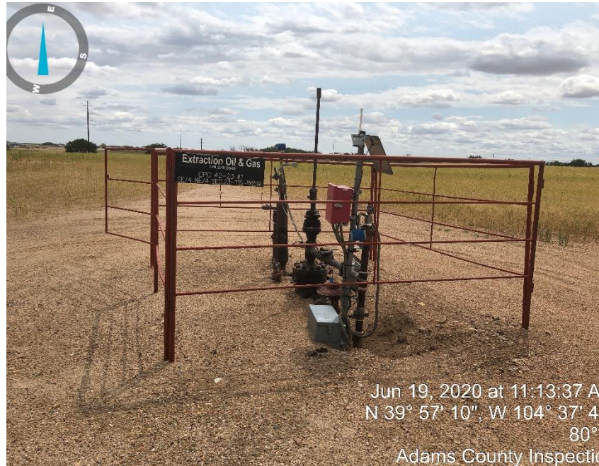
Photo #1 Well head.
