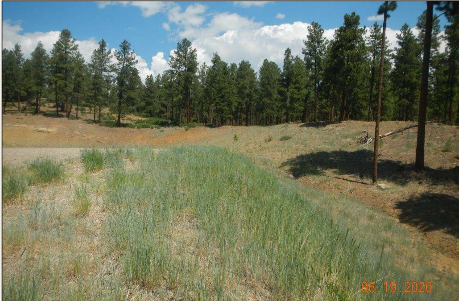
Photo 3. View of the northeastern fill slope from the northeastern corner facing westward.
