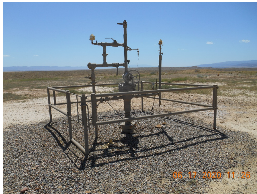
Wellhead with fence
