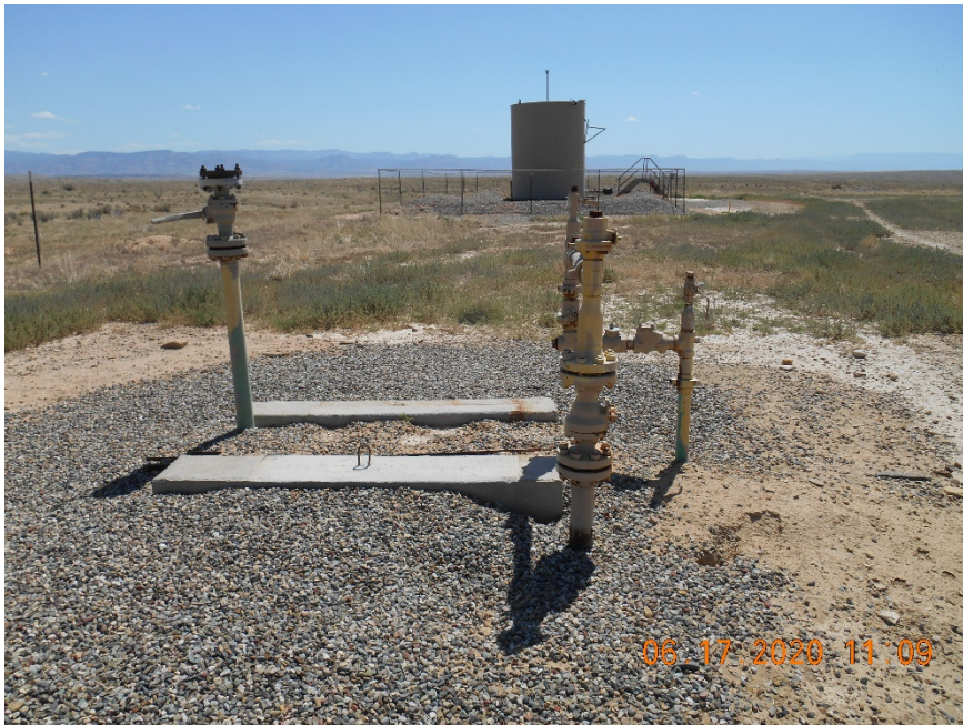
Separator risers locked out/tagged out
