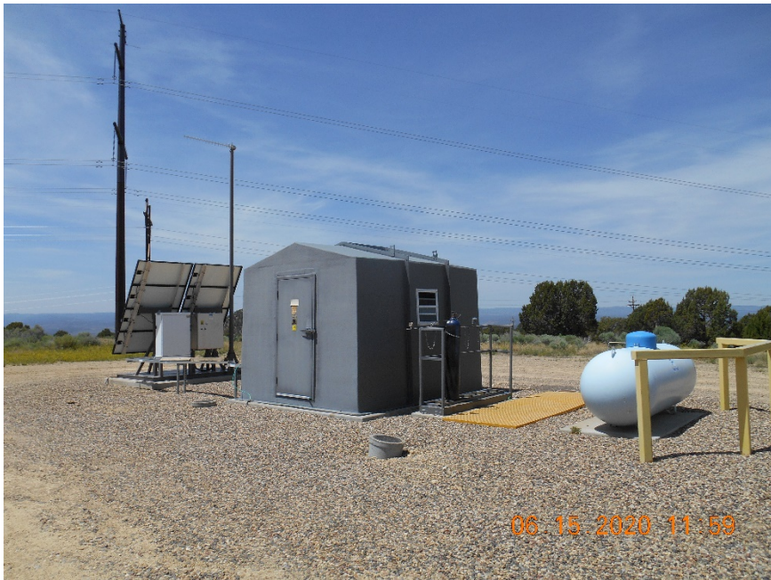
Injection wellhead inside housing
