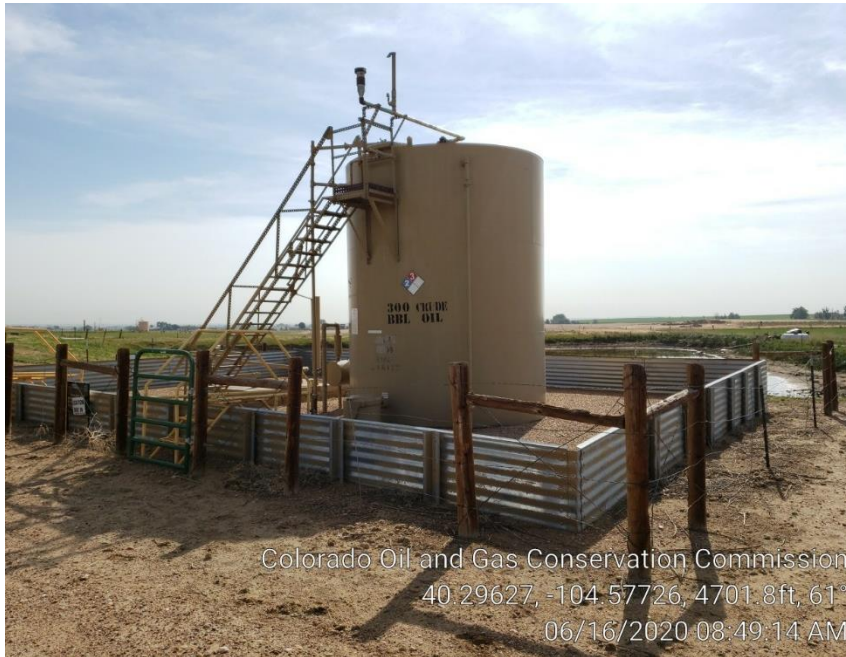
Photo #3 Tank Battery
