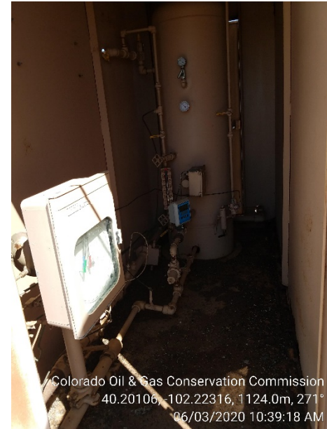
2. Gas meter and Vertical gas separator
