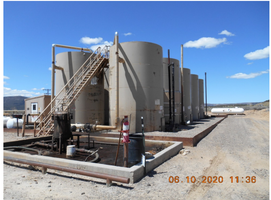
Tank battery and offload station
