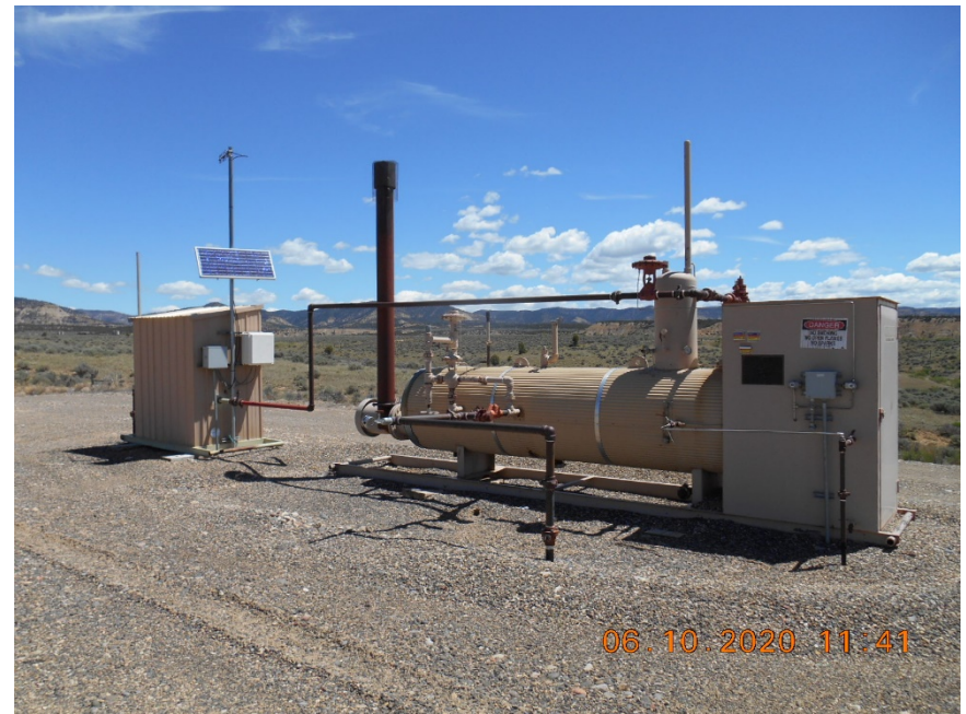
Separator and meter housing
