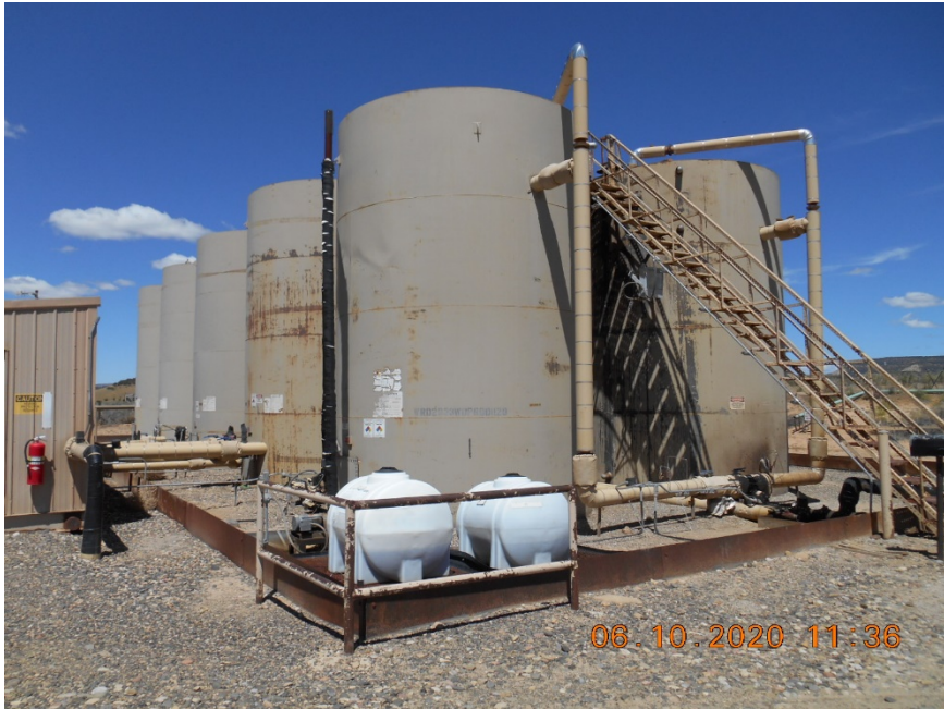
Tank Battery with secondary containment of chemicals
