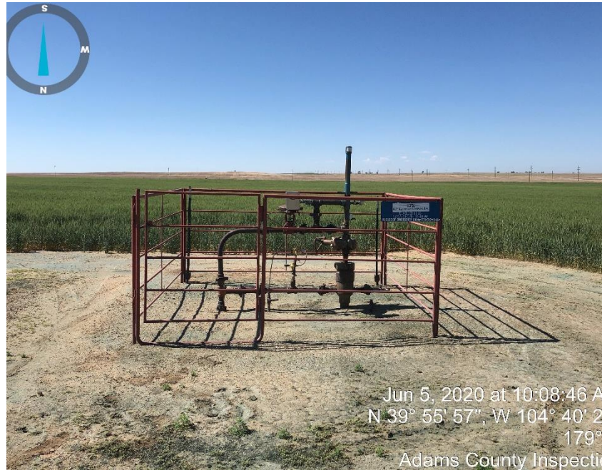
Photo #3 Well head.
