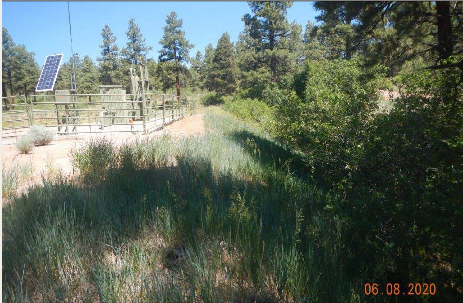
Photo 2. View of the eastern fill slope from the southeastern corner facing northward. Revegetation is progressing with western wheatgrass and rubber rabbitbrush.
