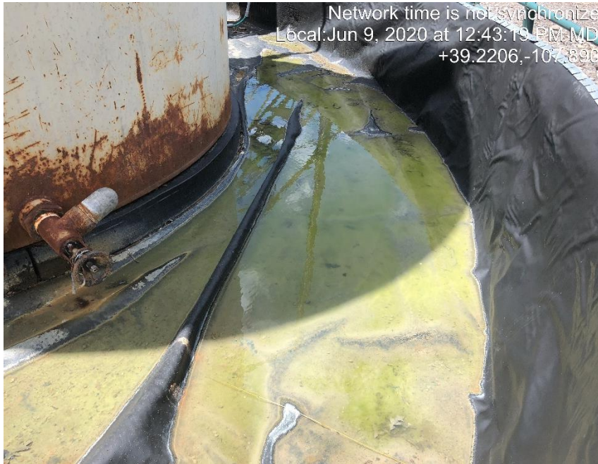
Photo #1332 Drain valve on tank #4-5 dripping condensate.
