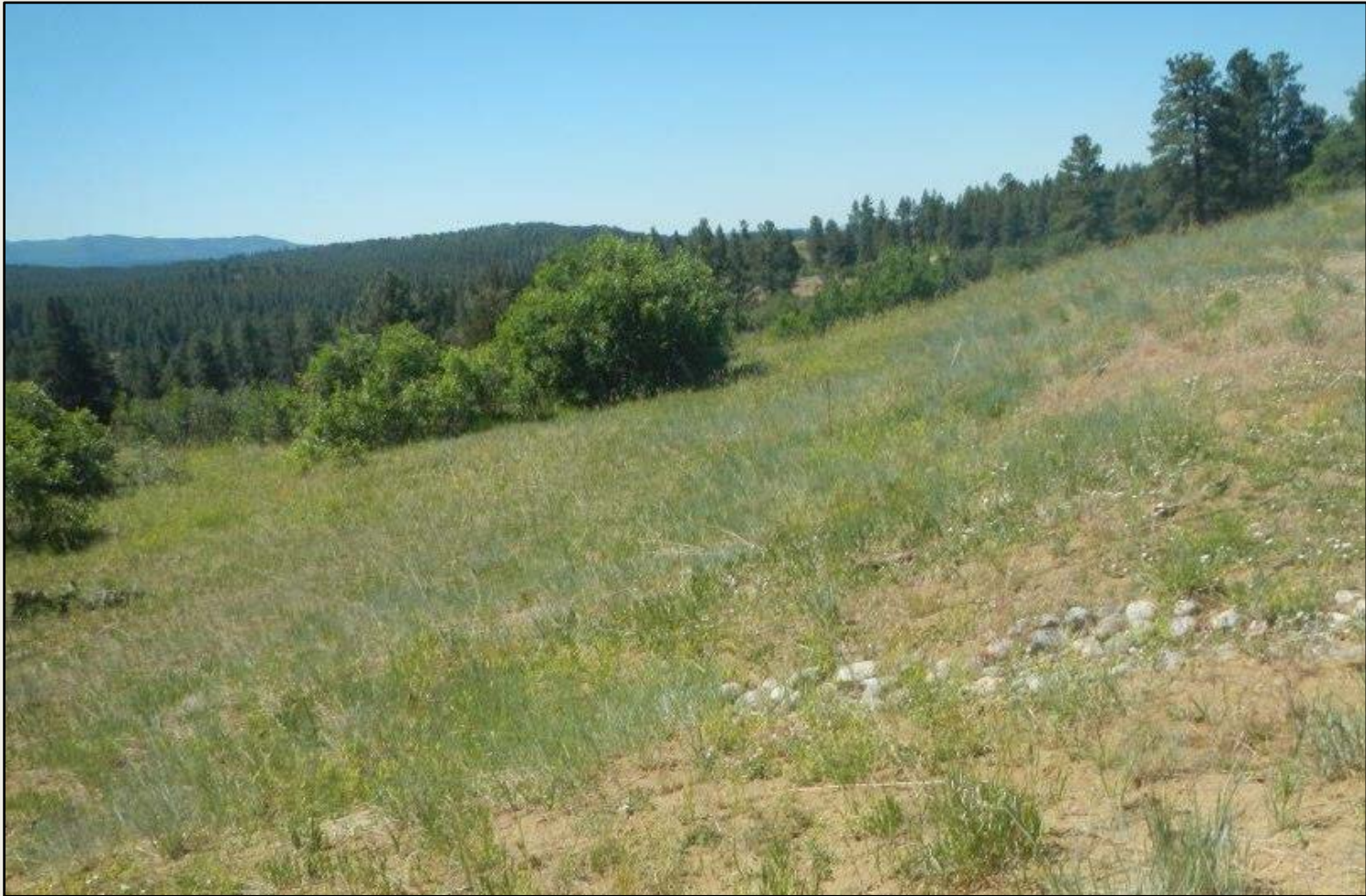
Photo 2. View of the eastern fill slope from the northeastern corner facing southward. Revegetation is progressing with grasses such as western wheatgrass and smooth brome.
