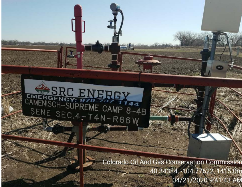
Wellhead sign on 4/21/2020
