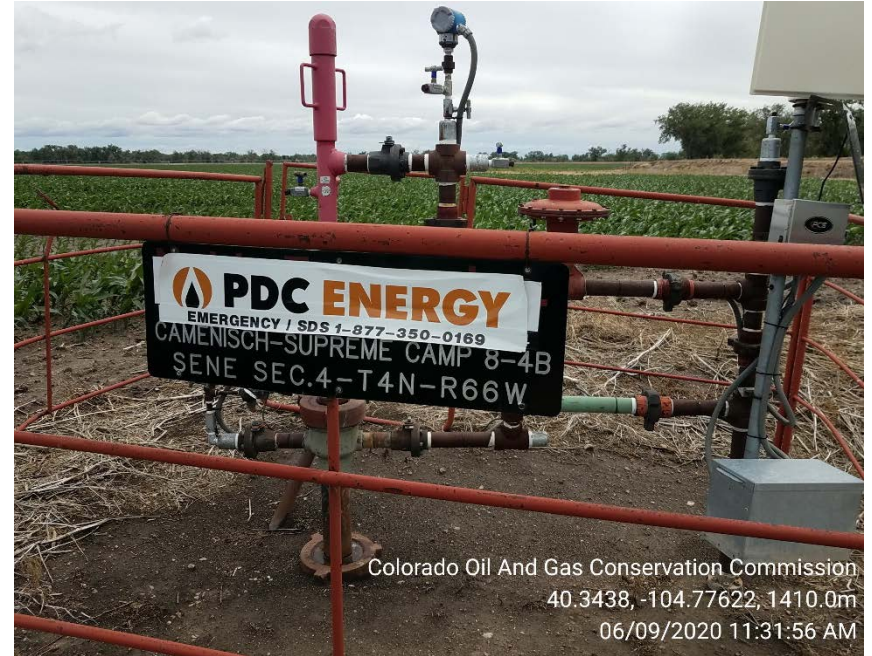
Wellhead sign on 6/9/2020
