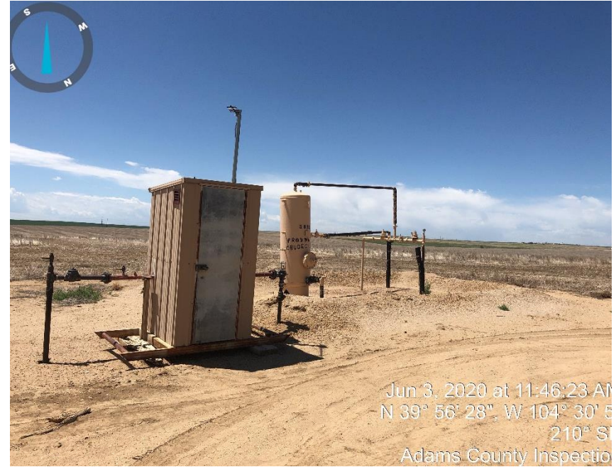
Photo #2 Meter and Separator.
