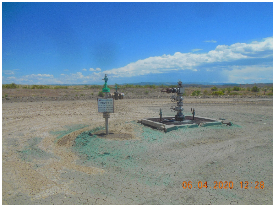
Injection wellhead. Temporarily abandoned.
