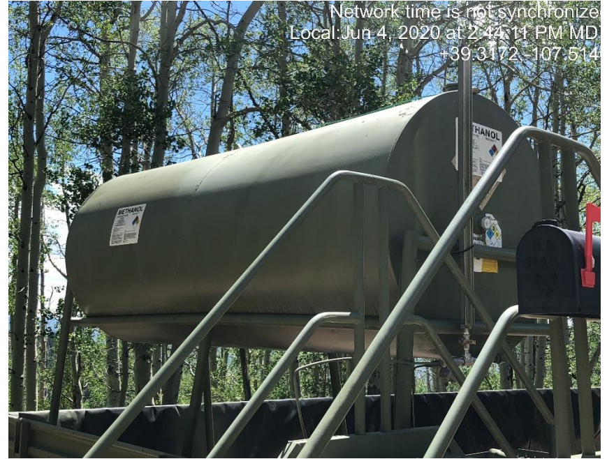
Photo #1318 Methanol tank not properly labeled.
