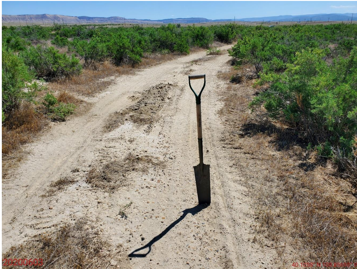
Photo 13: Photo taken from the southern section of the access road, facing east. Photo shows inspector tested for compaction along the access road with a 16 inch shovel; Inspector was unable to easily penetrate the soil surface of the access road; Compaction concerns remain.
