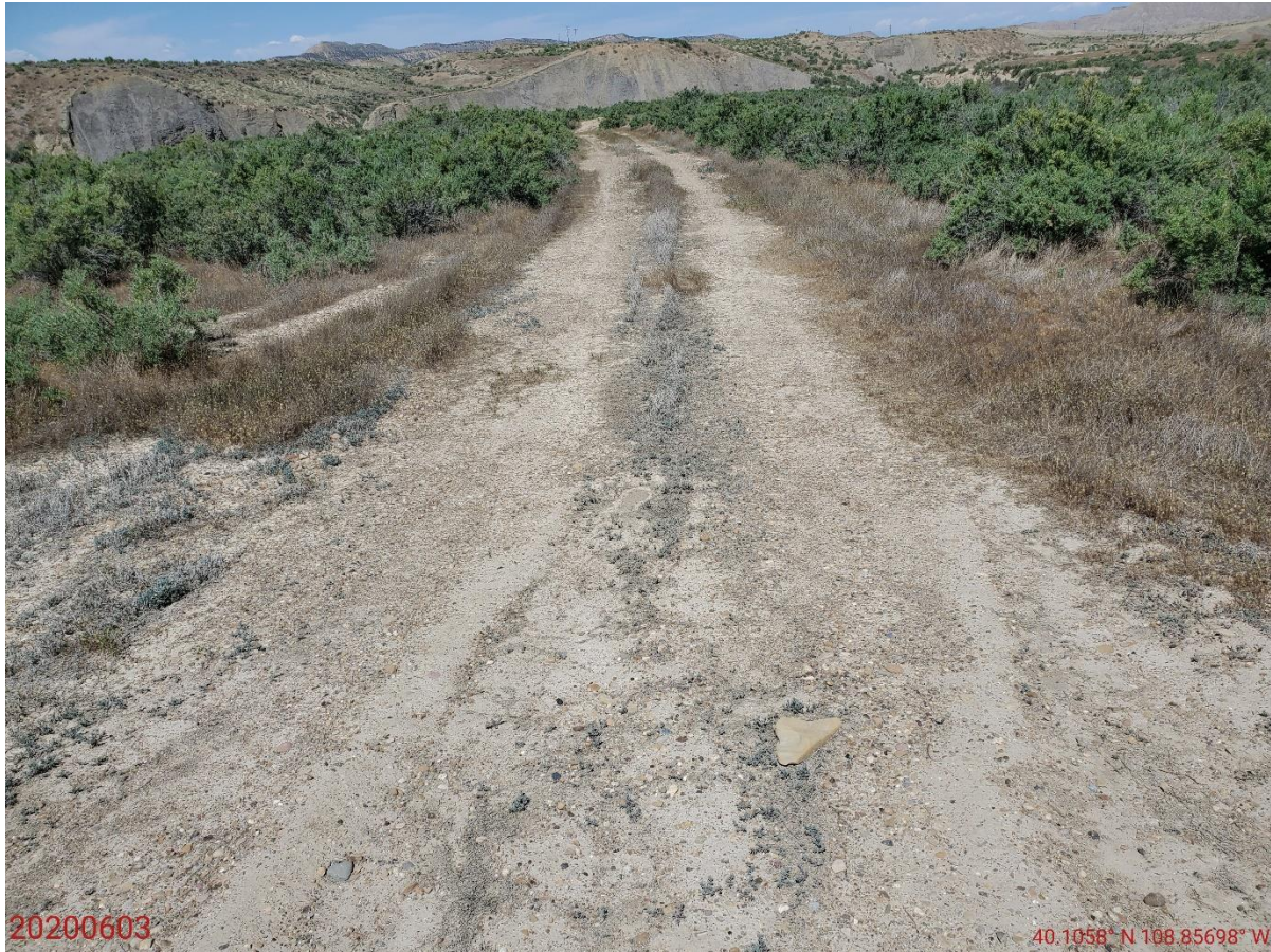
Photo 2: Photo taken from the northern portion of the access road, facing west. Unable to observe evidence that reclamation has been conducted on access road pursuant to 1004 Rules.
