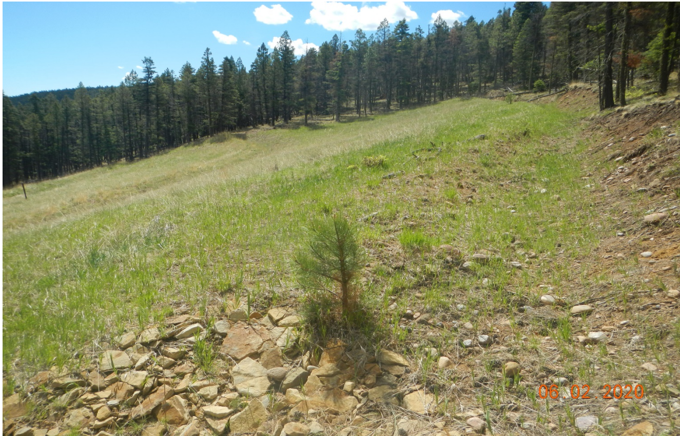
Photo 8. Facing southeast at the top portion of the location. There is a perimeter run-on ditch at the top portion of the location. This area should have been fully contoured into the terrain in order to fully reclaim this area.
