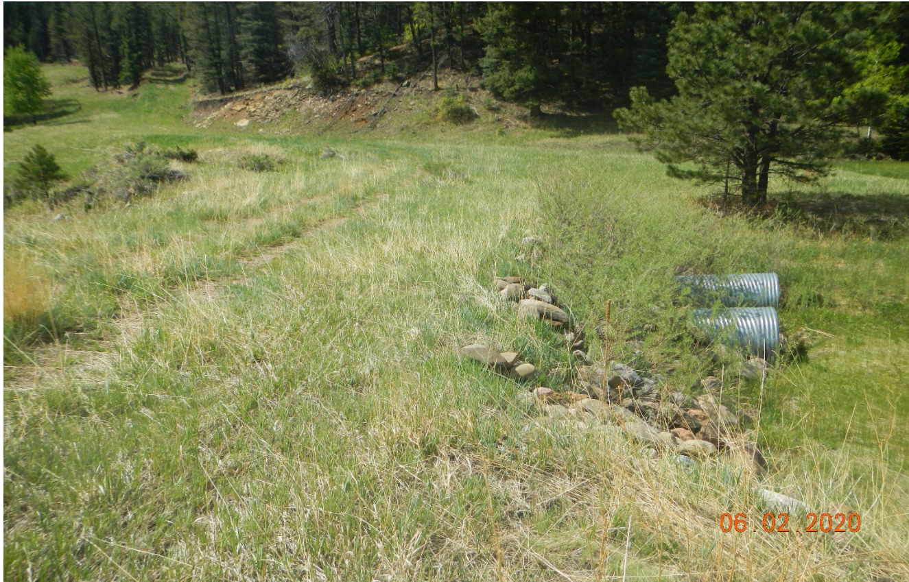
Photo 2. Facing south along the drainage crossing. There are two large culverts installed in the drainage crossing. There was no stormwater issues observed in this area.
