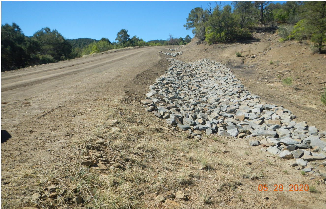
Photo 1. The erosion gully observed in previous inspection has been repaired and rock rip/rap has been installed.
