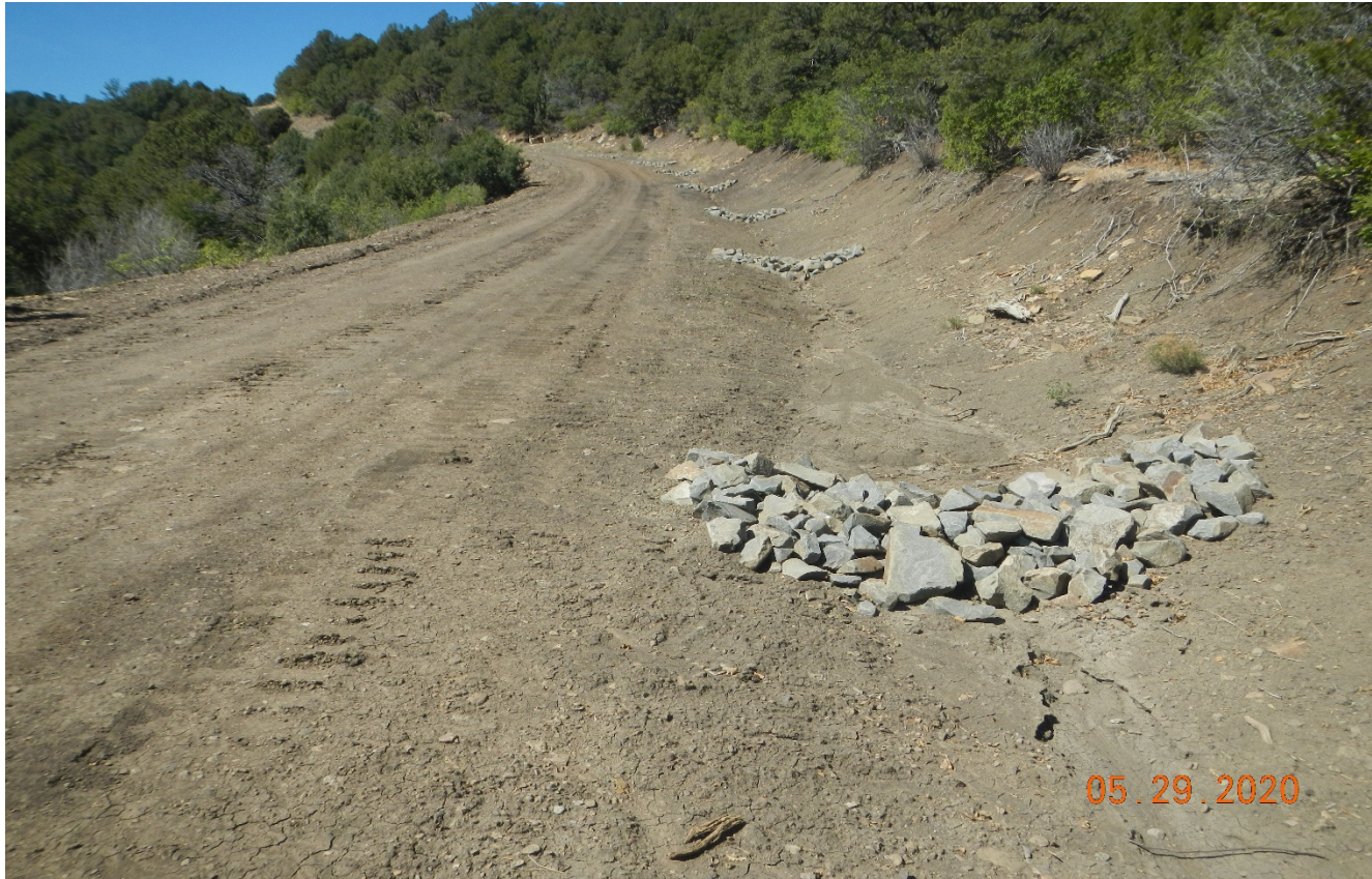
Photo 2. Facing southwest along the main road ascending the hill. Rock check dams have been installed along the road to the location.
